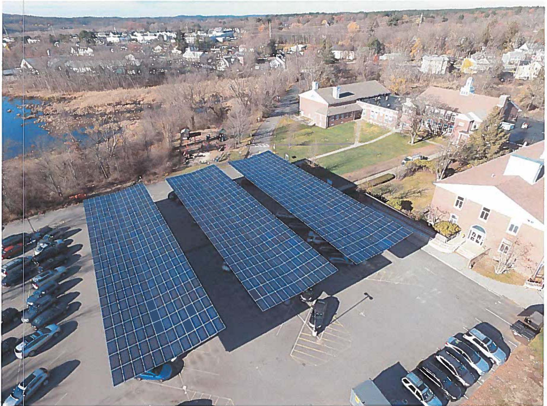
Wayland Town Building, System Type: Carport, Solar Panel Quantity: 825, DC Capacity: 260 kW, AC Capacity: 207 kW
