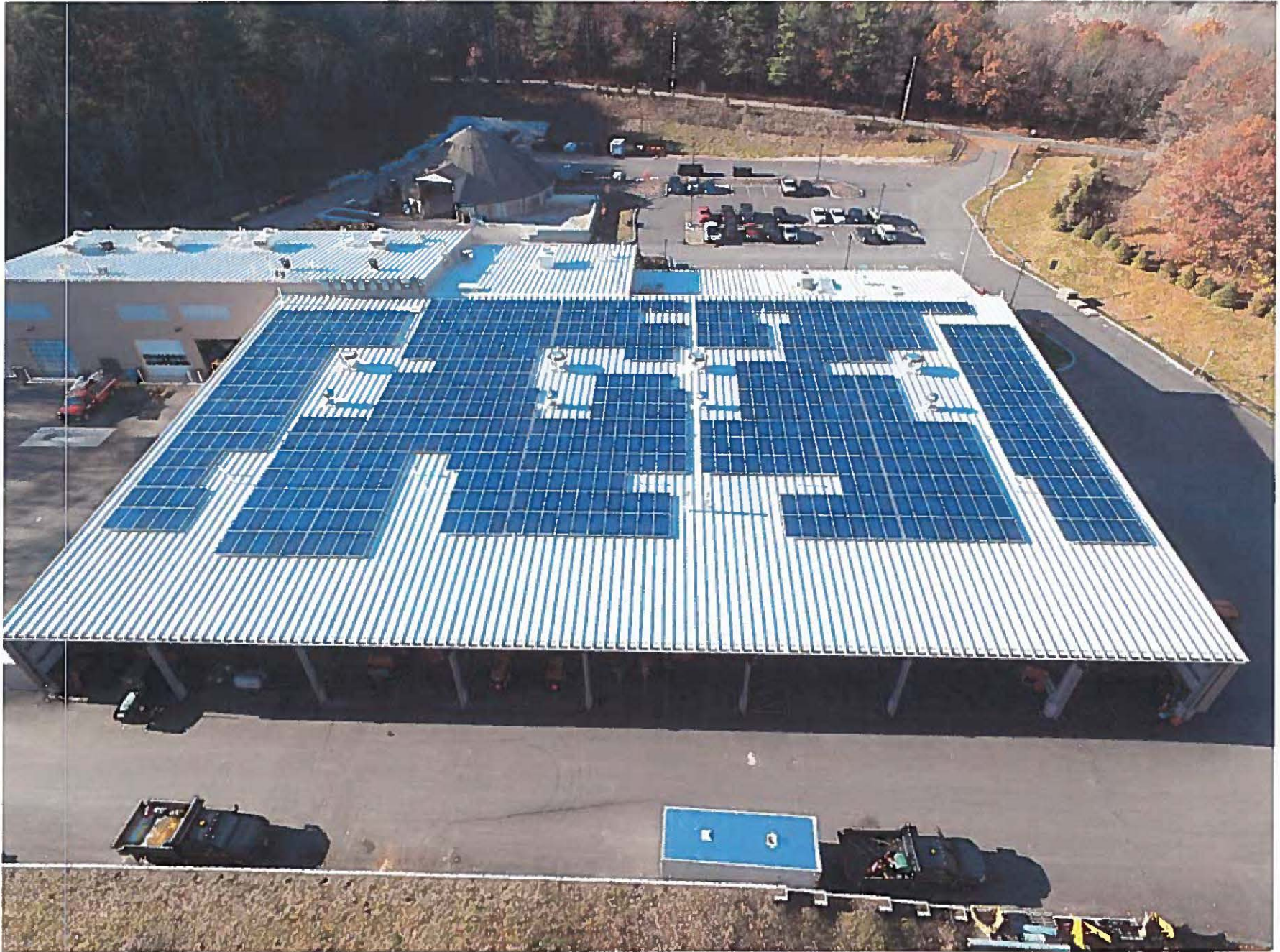
Wayland Department of Public Works, System Type: Rooftop, Solar Panel Quantity: 722, DC Capacity: 227 kW, AC Capacity: 176 kW
