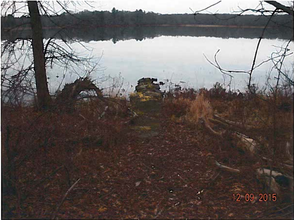
Existing Concrete Dock to be Removed and Replaced 5 Erwin Road, Wayland, MA
