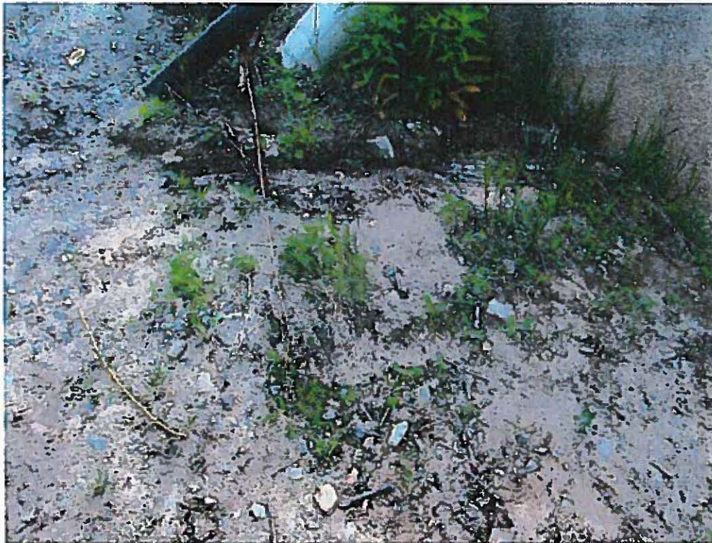
Photo 3: Example of minor erosion.
