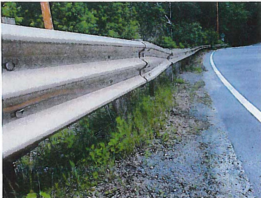
Photo 4: Northwest guardrail is set too high.
