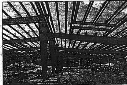
The steel structure goes up at the new Wayland Department of Public Works facility on River Road in Wayland. WICKED LOCAL PHOTO / DAN HOLMES
