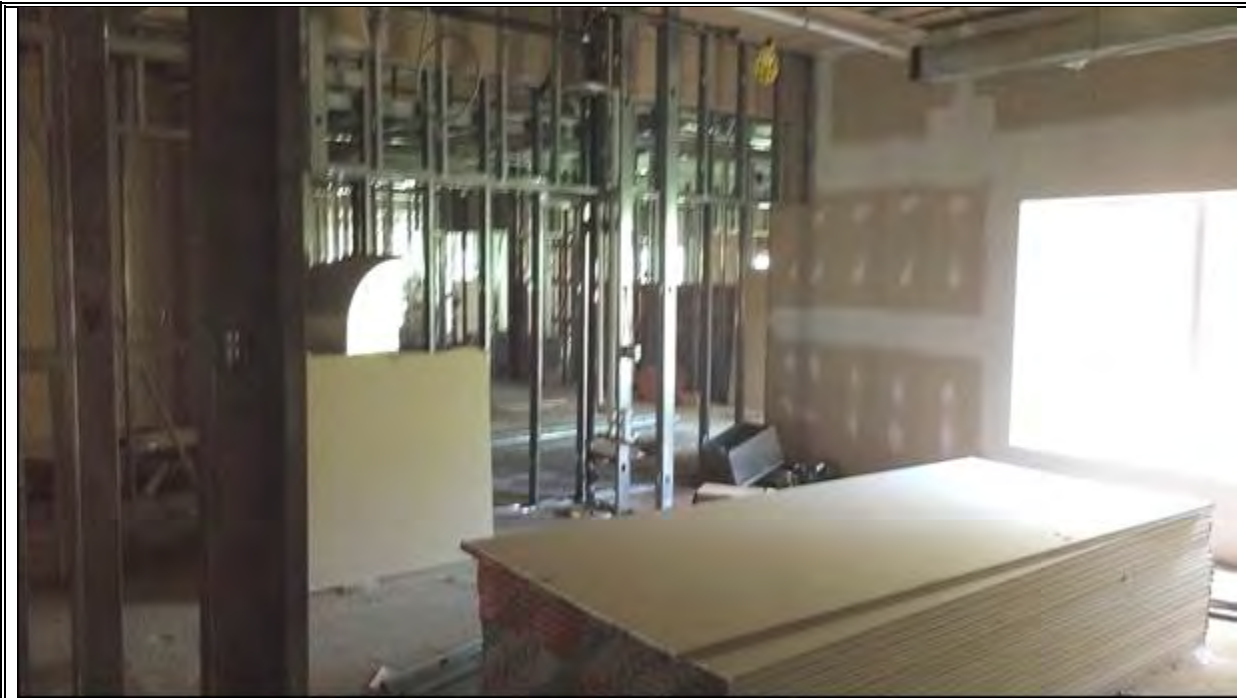
PHOTOGRAPH 3 UNFINISHED INTERIOR OF CURRENT SITE BUILDING. VIEW IS FROM MIDDLE OF BUILDING TOWARDS THE SOUTHEAST.
