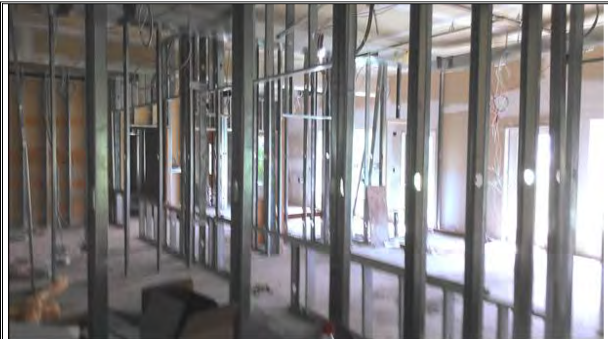
PHOTOGRAPH 4 UNFINISHED INTERIOR OF CURRENT SITE BUILDING. VIEW IS FROM EASTERLY END OF BUILDING TOWARDS THE NORTHWEST.
