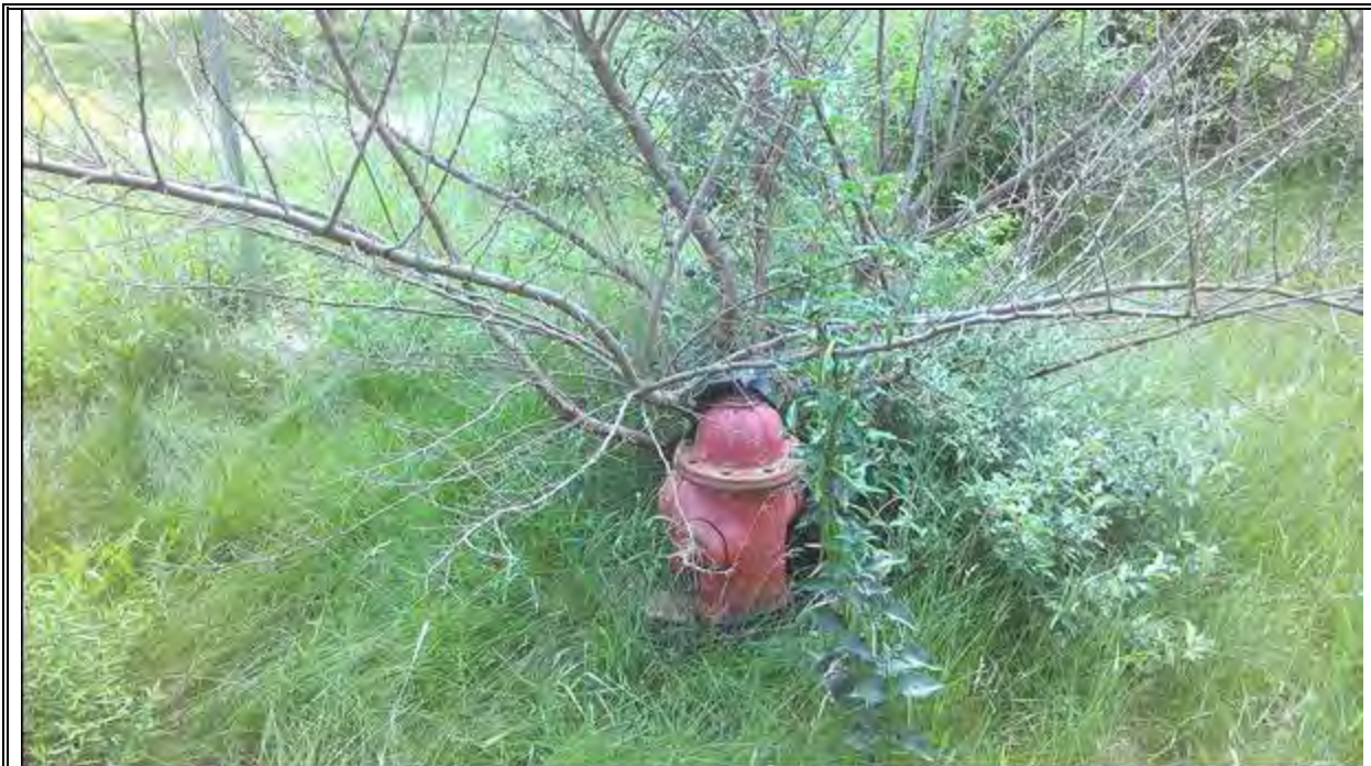
PHOTOGRAPH 8 OLDER HYDRANT CONNECTION IN OVERGROWN VEGETATION SOUTH OF BUILDING. VIEW IS TO THE SOUTH.
