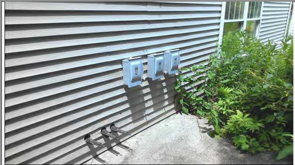
PHOTOGRAPH 7 STUBBED-OFF UTILITY CONNECTIONS ON SOUTHEAST BUILDING EXTERIOR. VIEW IS TO THE NORTH.
