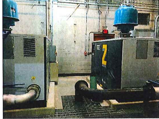
New Aeration Blowers 02/2019
