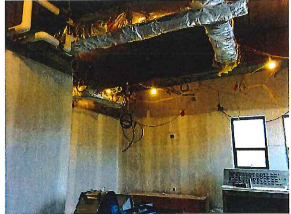
Admin. Building Control Room 02/2019
