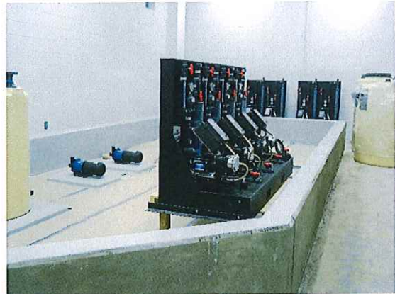
Admin Building New Chemical Metering 11/2018
