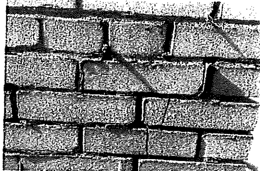
Defect #11 – Close-up photo of det. joints
