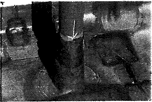
Defect #10 – Void in sealant at pipe flashing
