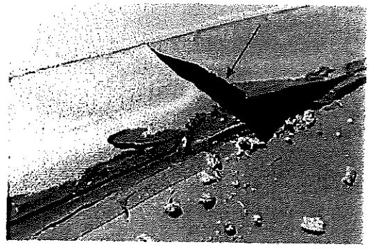
Defect #2 – Splits in EPDM batten strips
