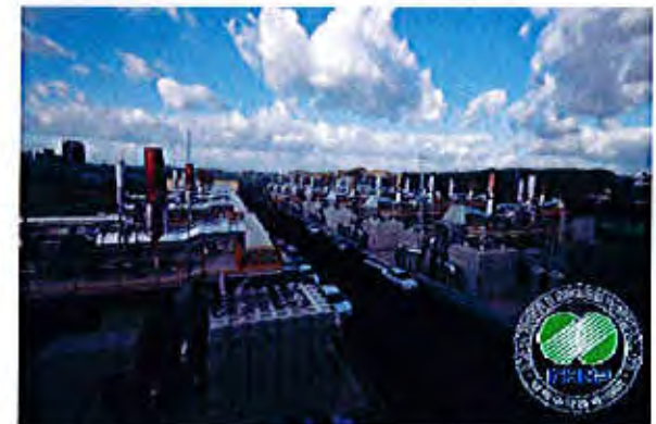
59 MW District Heating Fuel Cell in Seoul, Korea
