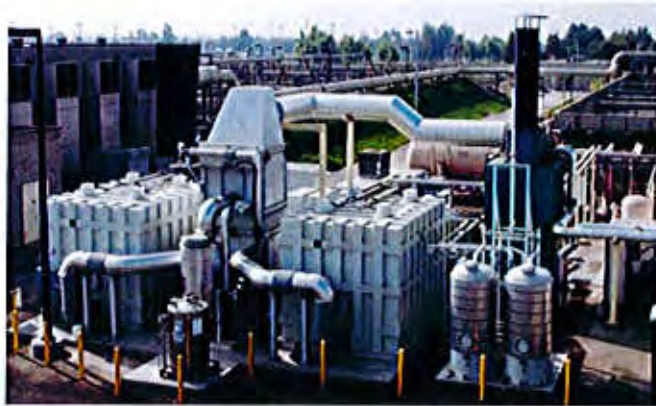
2.8 MW On-Site Biogas Fuel Cell in California
