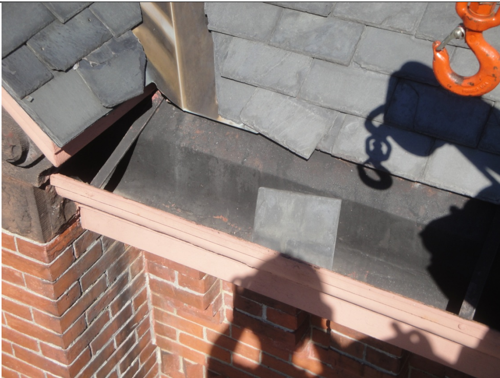
Photo R16 08/13/15 Photo Location: Valley of front dormer roof.
