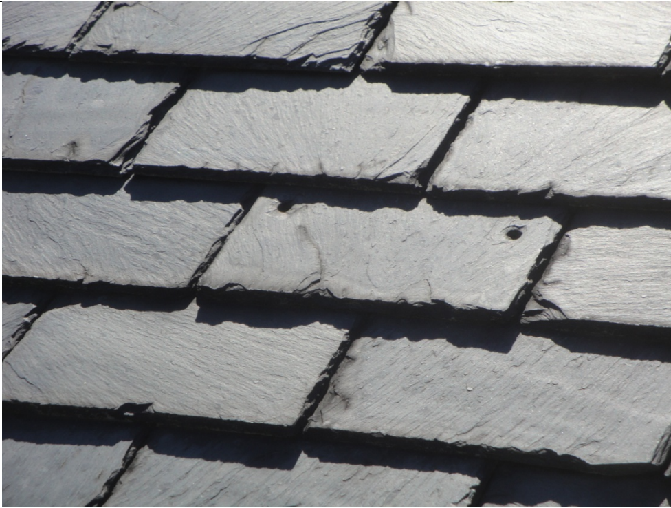
Photo R7 08/13/15 Photo Location: Upper main roof. Description: Typical original Monson slate on main roof.
