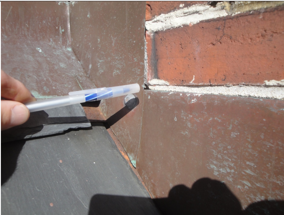
Photo R8 08/13/15 Photo Location: Low front entrance roof. Description: New red copper counter flashing and step flashing at roof to wall intersection. Note: void in masonry joint at new work.
