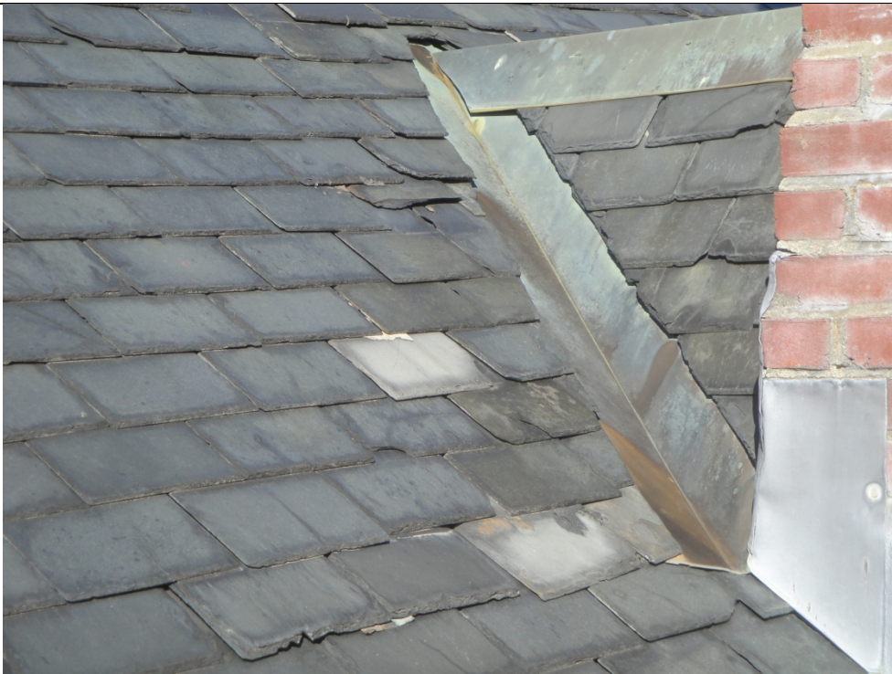
Photo R22 08/13/15 Photo Location: Upper main hip roof adjacent to remaining chimney.
