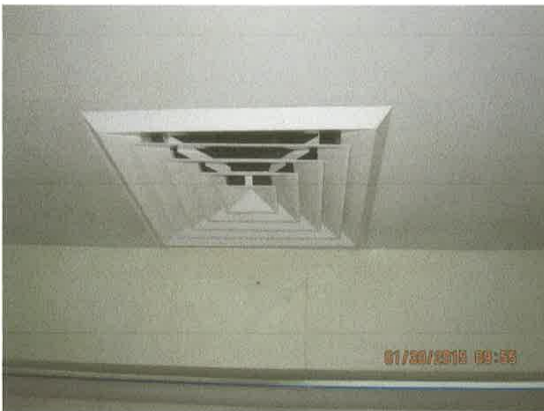
Photo 3 HVAC vent where leakage came through.
