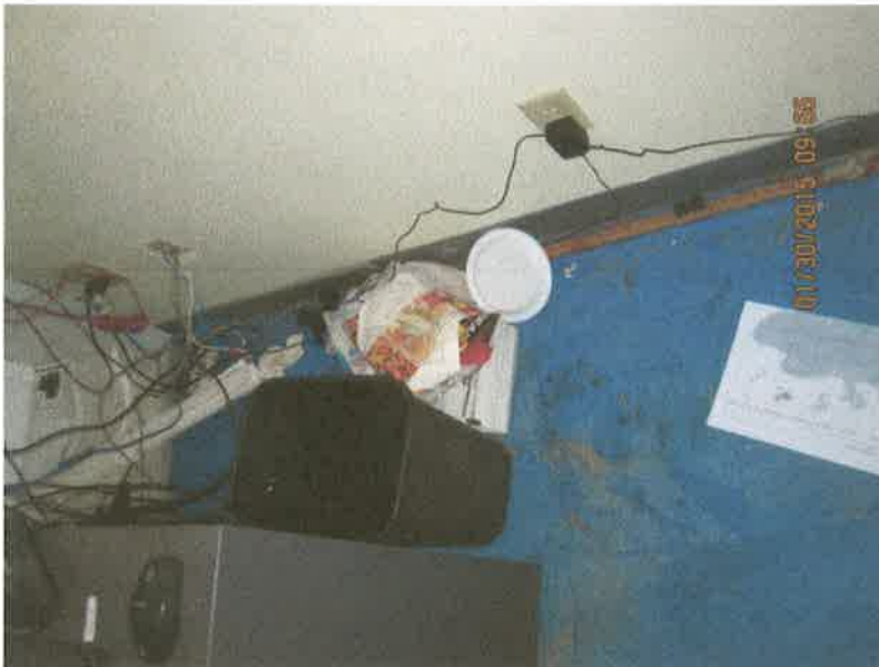
Photo 2 Office leakage area.
