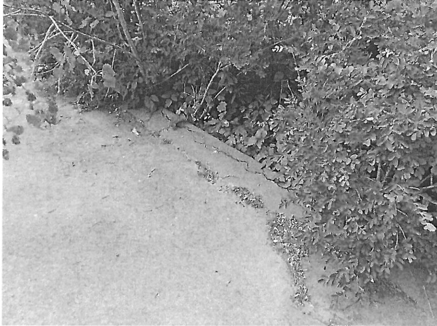
Cracked Bituminous Berm
