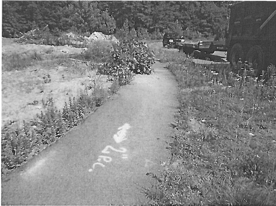
Overgrown Areas (Pine Meadow Road)
