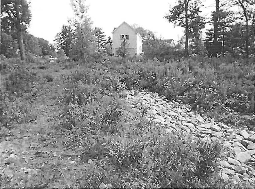
Overgrown Detention Basin
