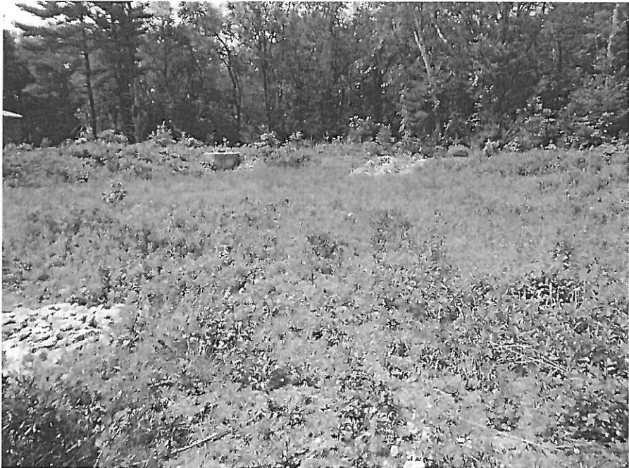
Overgrown Detention Basin
