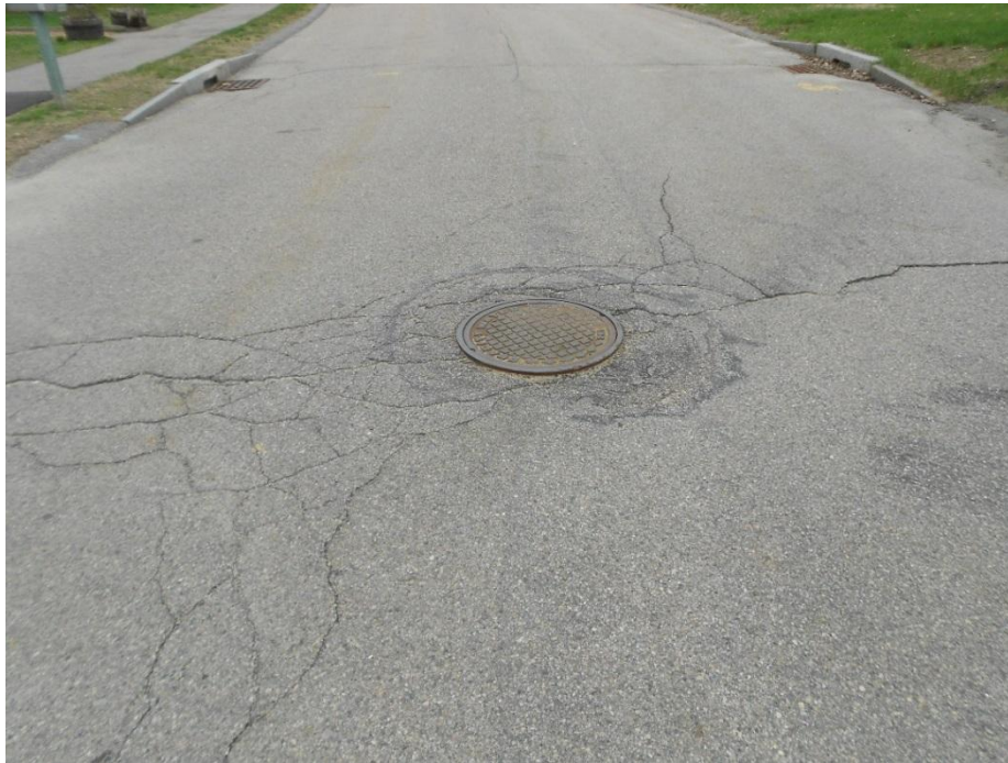
Incorrect Sewer Cover/Casting
