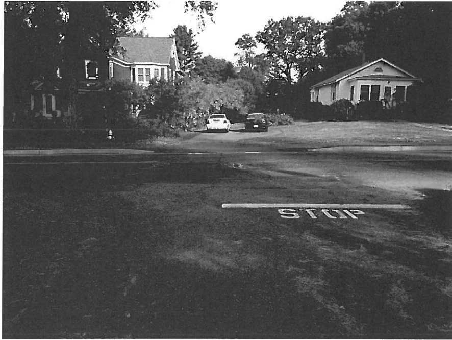
Village Street Water Trench Patch Damage
