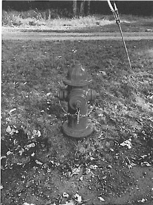
Installed Hydrant (Repaint/Flag per Town Standard)
