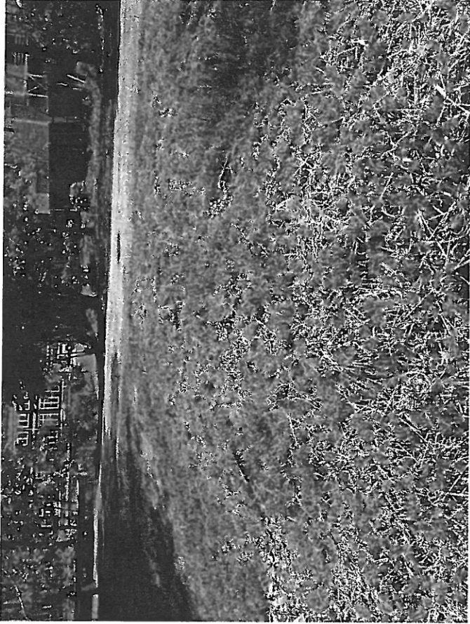
No level spreader or spillway on Basin 2
