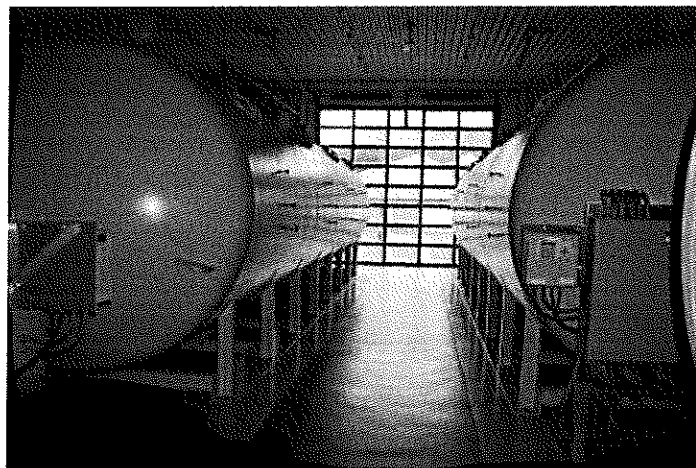
Figure 1 Pressure Filter Vessels (Natick, MA)
