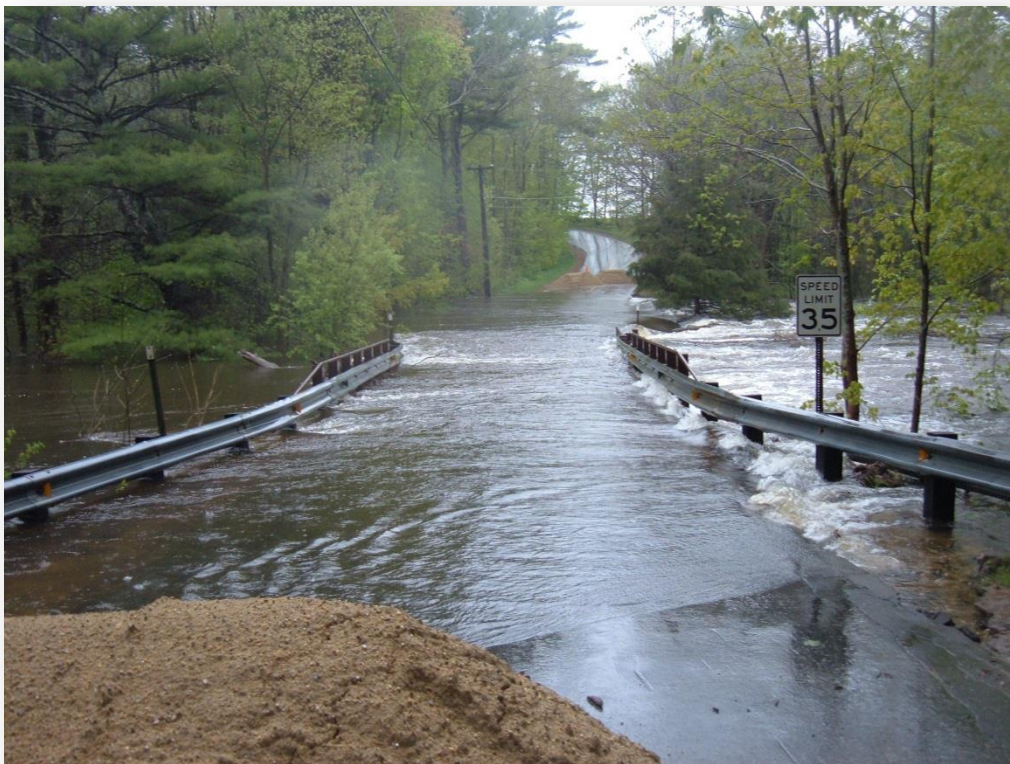
High Road Bridge, May 2006 Flooding Event
