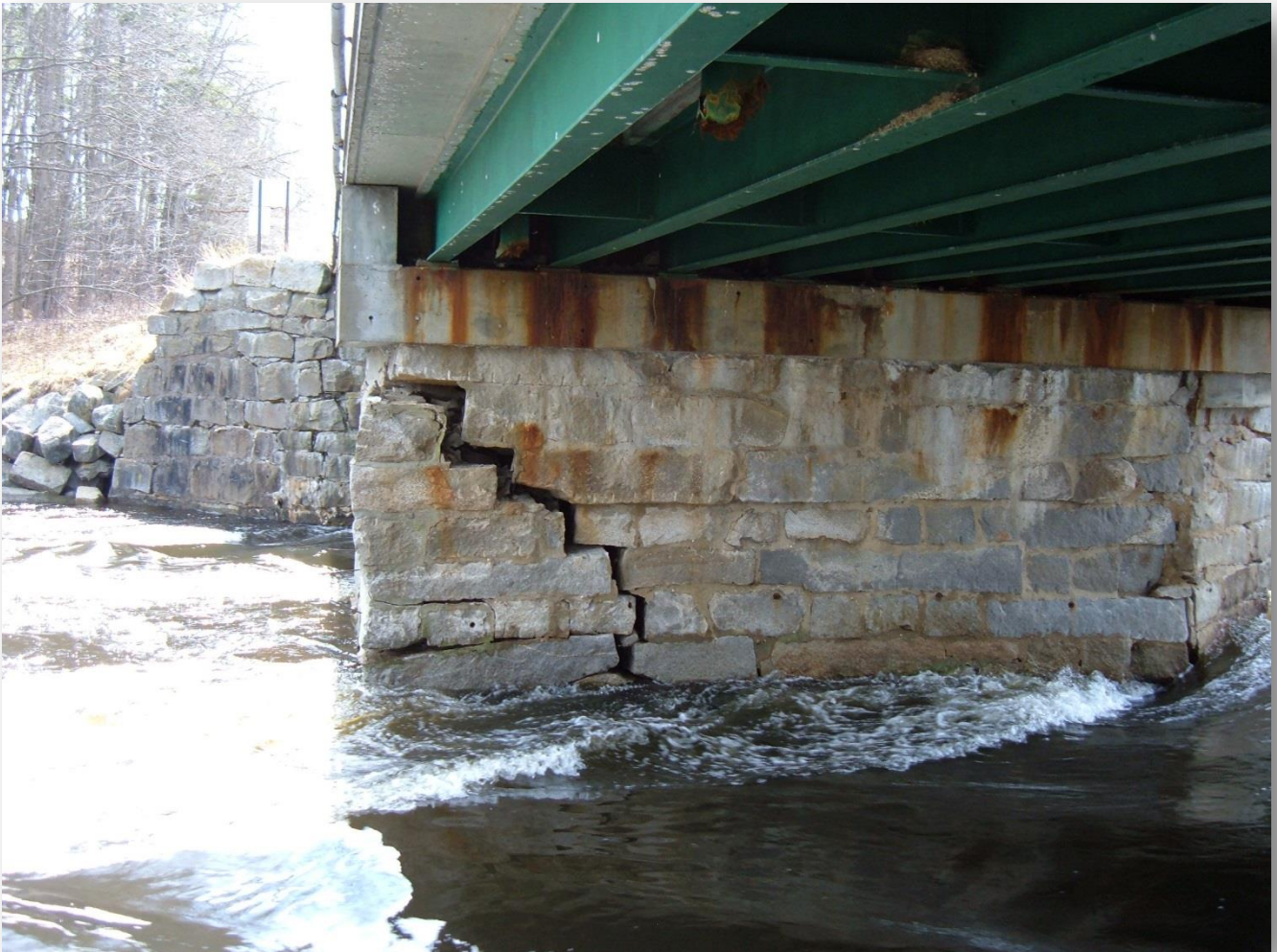
Damage to Lee Hook Road, Flooding
