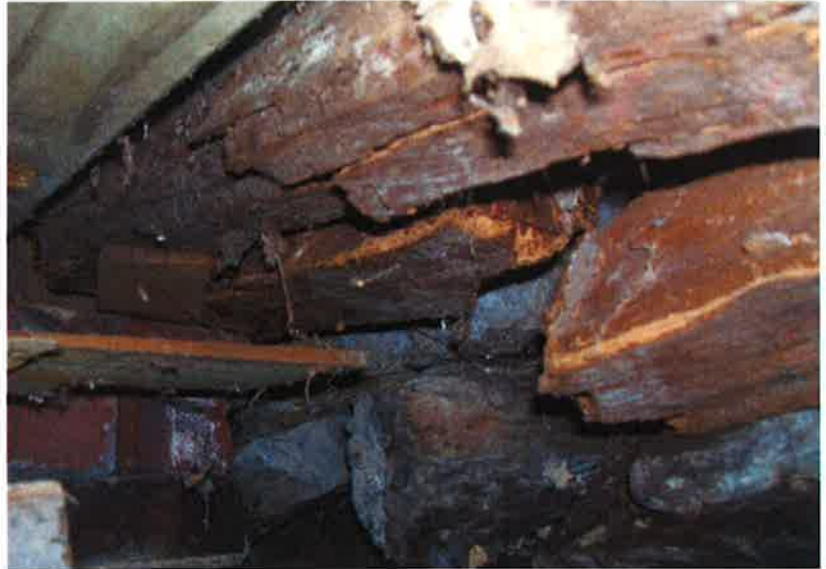
Figure 3 The wood structure under the floor has not survived its 171 years in the same condition as the brick exterior.
