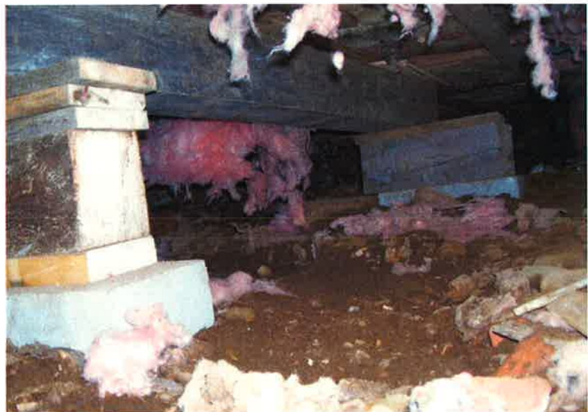
Figure 4 The dirt floor in the crawlspace has no vapor barrier and only limited ventilation leading to the deterioration of the wood structure. Uninsulated areas of the floor can be seen at the top of the photo. Columns of concrete blocks have been added to support the beams under the floor.
