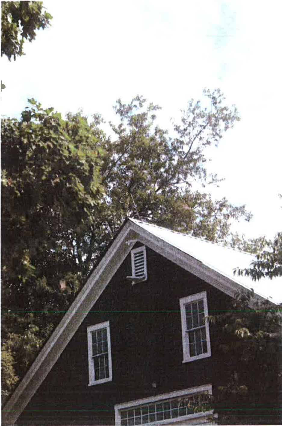
Detail front of barn including glassed lightning rod and offset of front door to match uneven bays of 14' ,12'nd 12' roof pitch is approx. a 9/12.
