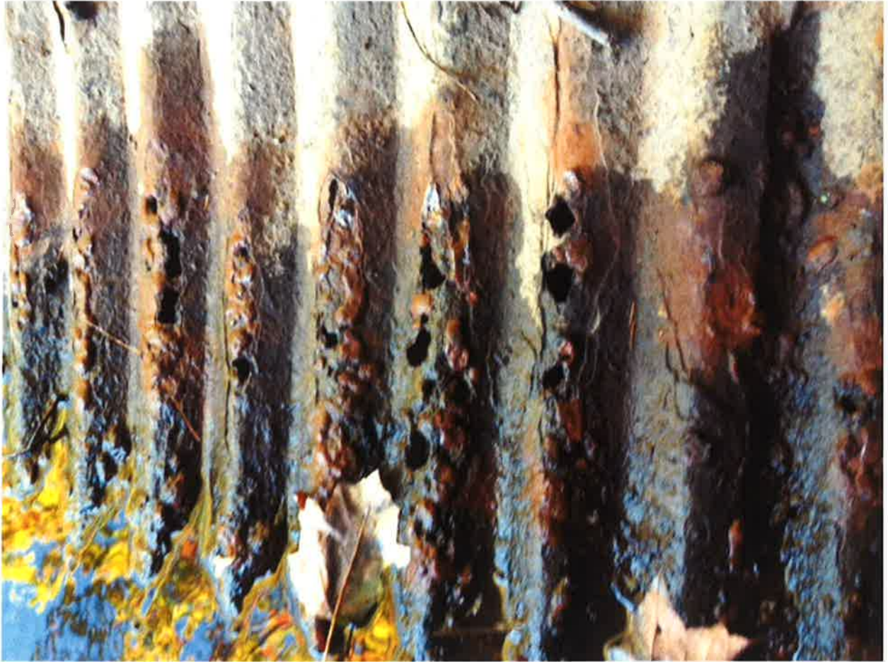
Rusted holes in the invert of the Tuttle Rd Culvert
