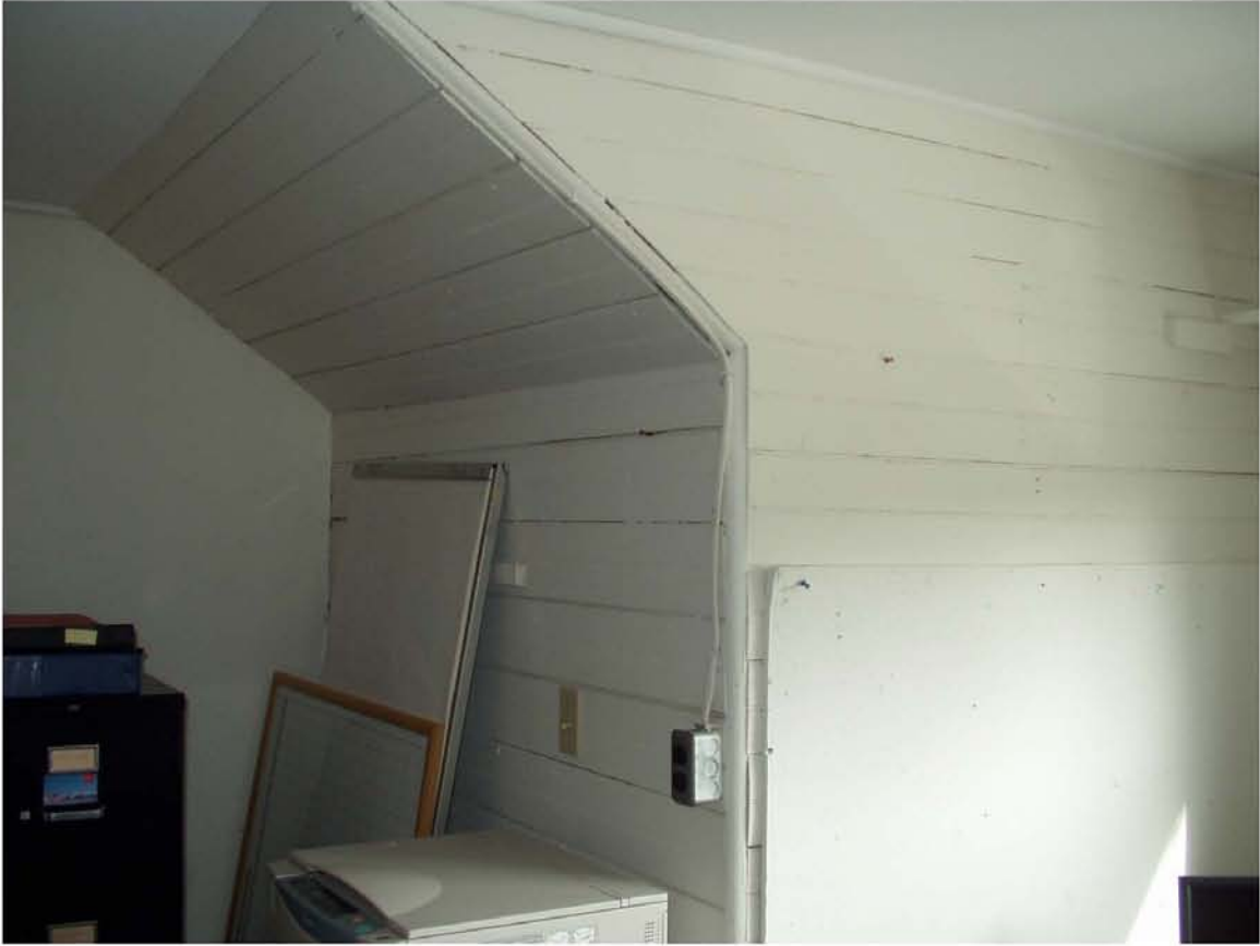
TOWN HALL ILLEGAL WIRING AND CABLING BEHIND AIR GRILLE
