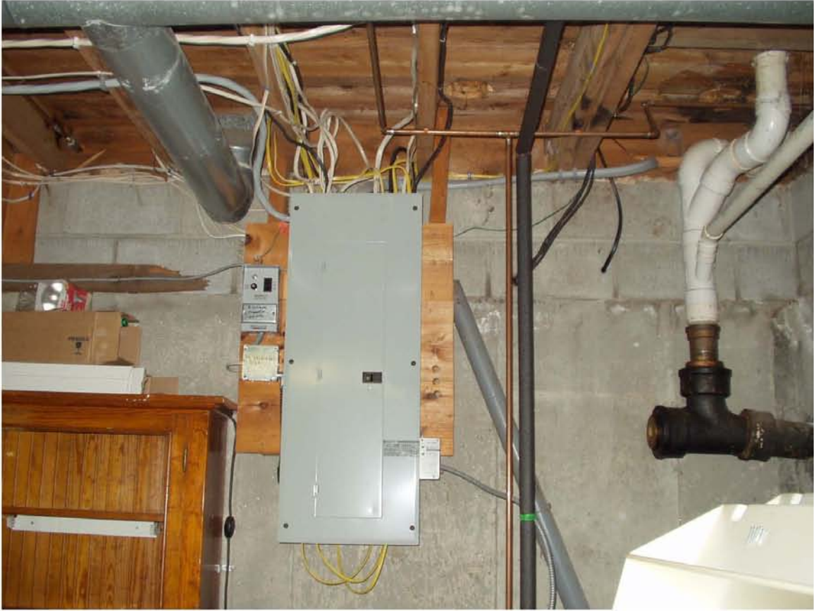
LIBRARY BASEMENT SUB PANEL
