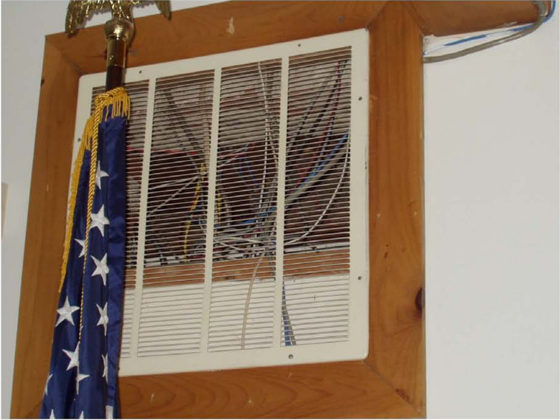
TOWN HALL ILLEGAL WIRING AND CABLING ALONG HEAT PIPES EXPOSED
