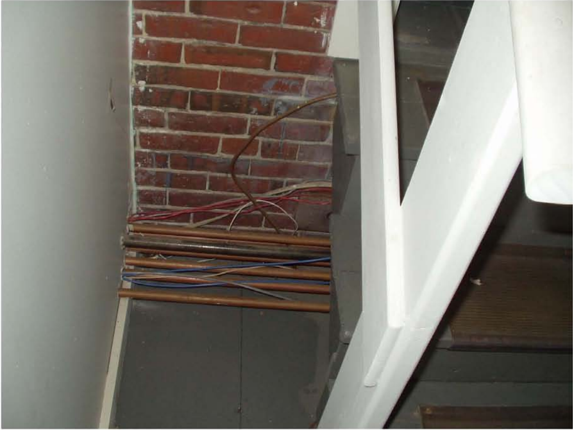
LIBRARY MAIN PANEL WITH TRANSFER SWITCH ON LEFT FOR EMERGENCY GENERATOR TO HEATING CIRCUIT
