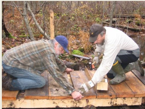
TOM LEE AND LORNE FITCH (A VISITING FRIEND FROM ALBERTA) BUILDING A BRIDGE IN THE TOWN FOREST IN 2009
