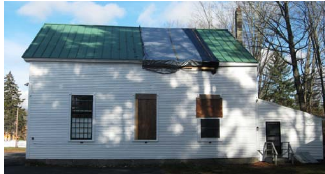
Jeremiah Smith Grange, Lee NH damaged by Hurricane Sandy.
