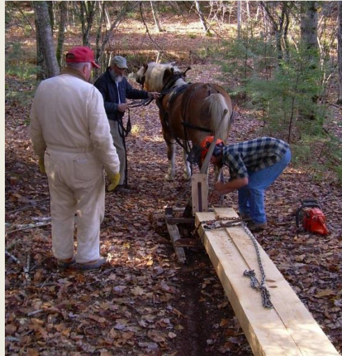
CLYDE FOGG, CHUCK COX AND JOEL MILLER ATTACHING BEAMS FOR HAULING TO SITE IN 2009
