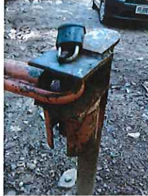
Pipe gates locks
