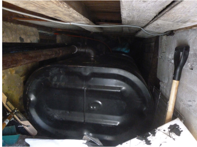
OIL TANK UNDER PORCH
