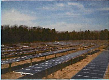
3 MW Delsea Vineland, New Jersey
