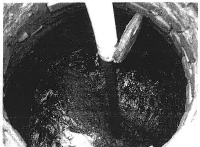
60 Discharge During Cleaning
