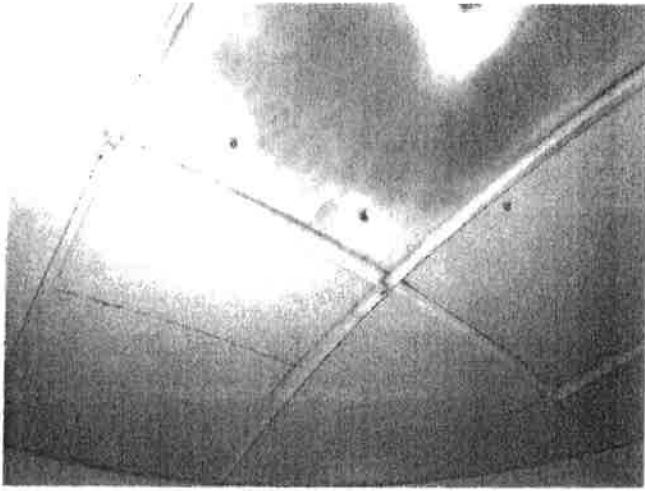
55 Overhead Panels Yielding Expired Coating And Blotch Rusting
