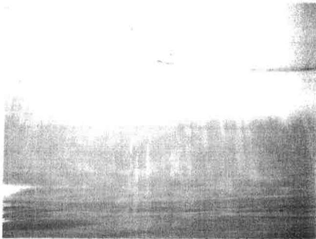
51 Interior Walls Found With Coating Failure, Exposed Steel, Corrosion, Pitting And Staining
