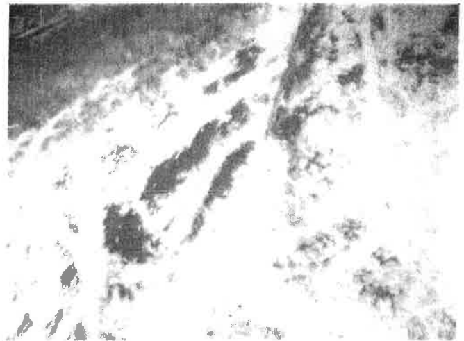
28 Floor Panels Found Yielding Heavy Staining After Cleaning
