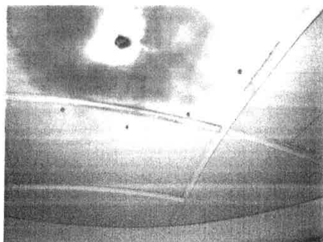
54 Overhead Panels Yielding Expired Coating And Blotch Rusting
