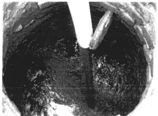
60 Discharge During Cleaning
