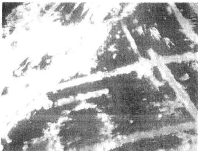
29 Floor Panels Found Yielding Heavy Staining After Cleaning
