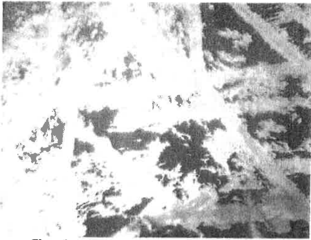
31 Floor Panels Found Yielding Heavy Staining After Cleaning
