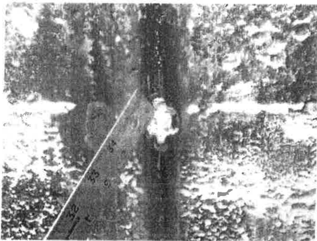
47 Interior Walls Found With Coating Failure, Exposed Steel, Corrosion, Pitting And Staining
