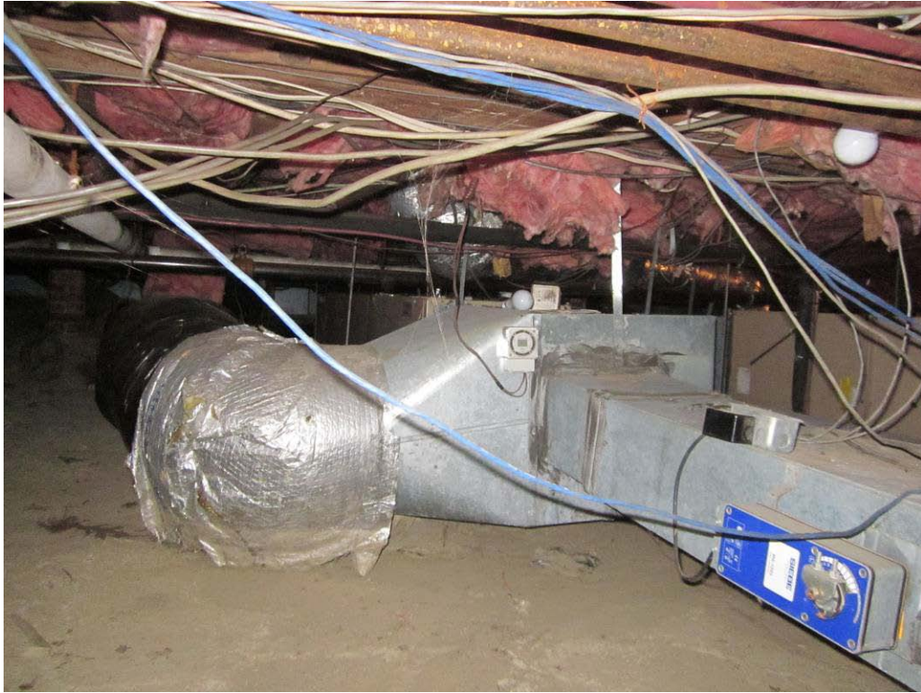
Photo 7 - Crawl space abandoned mechanical equipment
