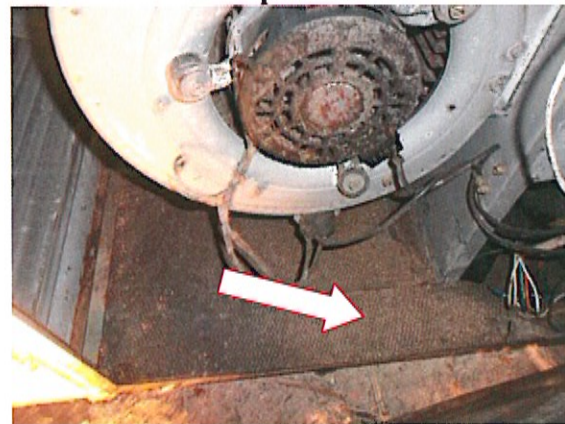
The AHU appears to have soils within the unit, likely from high water levels
