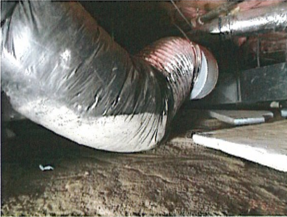
Visible indication of high water mark on ductwork, level is higher than AHU units
