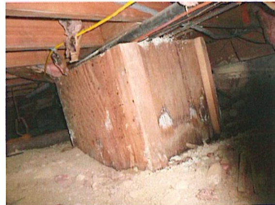
Plywood forms around steel posts have visible heavy mold growth
