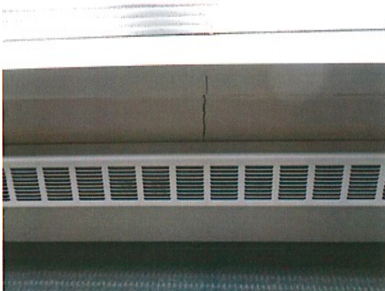
Council Chambers with a crack in south side exterior wall below the window
