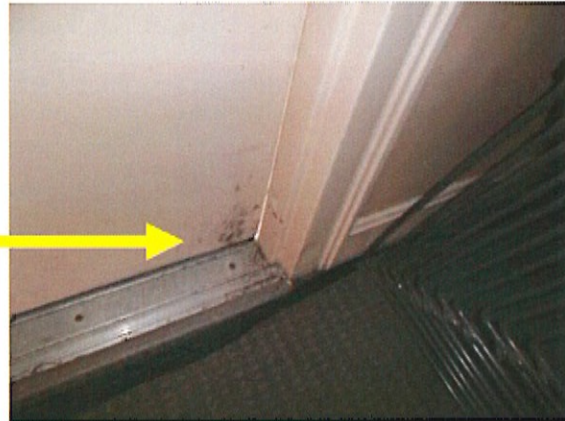
A large gap in the Chambers Room door with visible mold growth for door surface
