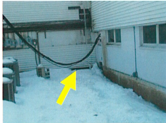
Window appears to be an access point for water and rodent intrusion
