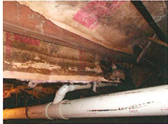
The paper faced insulations are moldy, moisture damaged, and have rodent urine
