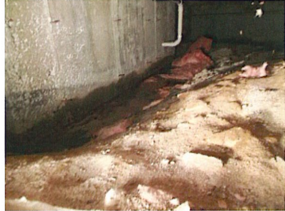
Standing water around base of elevator shaft in crawl space
