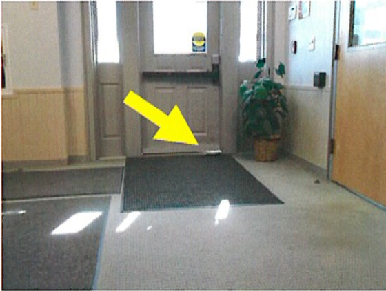
Door sweep gap allows for rodent/insect access and exhaust fume infiltration
