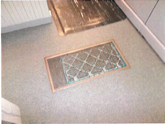
Ventilation return in floor for original structure level one – north side
