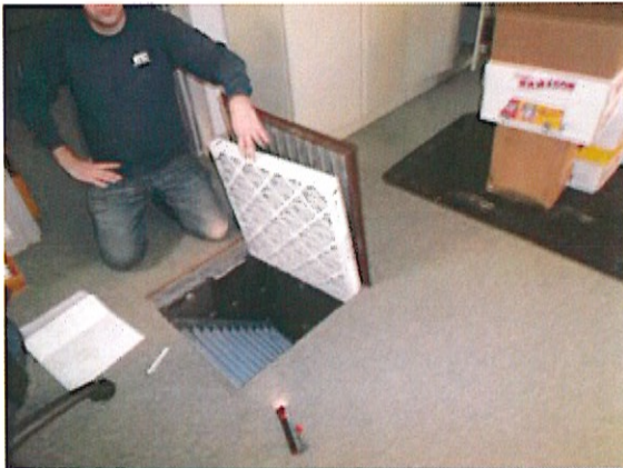
Ventilation return in floor for original structure level one – south side
