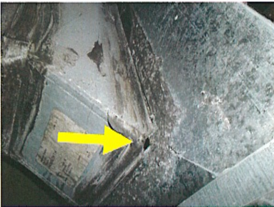
One of several locations with unsealed holes in ventilation ductwork
