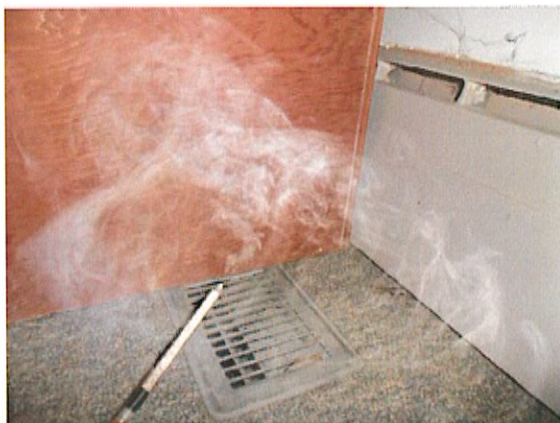
Passive air movement out of non-operating ventilation supply floor vent
