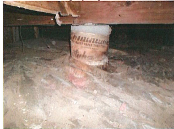
Sonotubes within the crawlspace have visible mold growth
