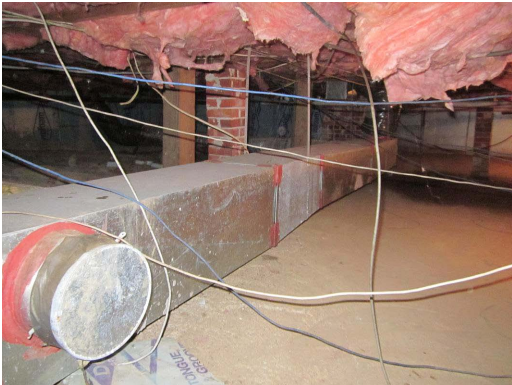
Photo 6 - Crawl space abandoned mechanical equipment
