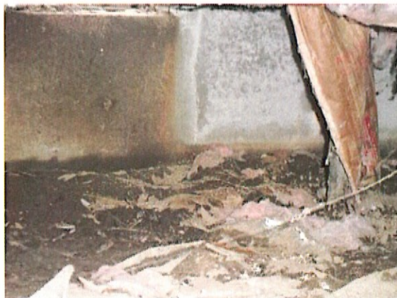
Soils below window above show signs of routine water intrusion
