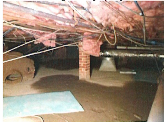
Settled damp soil covers the cement floor area at west end of crawlspace
