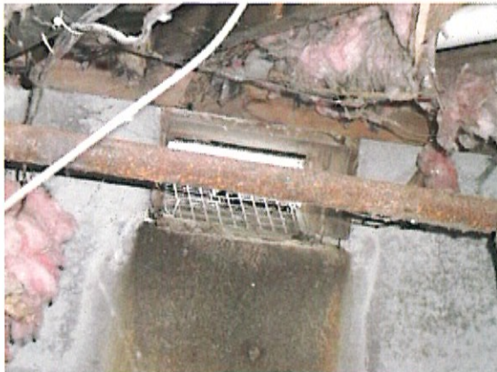
This window appears to allow water and rodents access into the crawlspace
