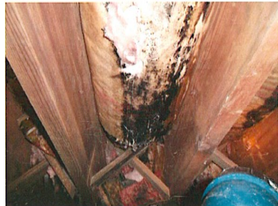
Insulation damage due to crawlspace humidity, mold growth and rodent urine
