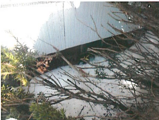
Snow accumulations covering crawlspace windows
