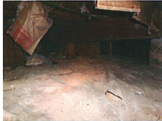
The east end of the crawlspace (add-on structure), has damp/wet sand floor with a tattered poly vapor barrier
