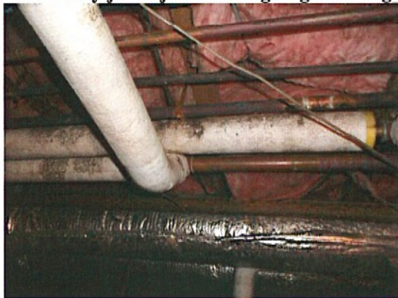
Mold growth covers much of the paper covering for fiberglass insulations in crawlspace
