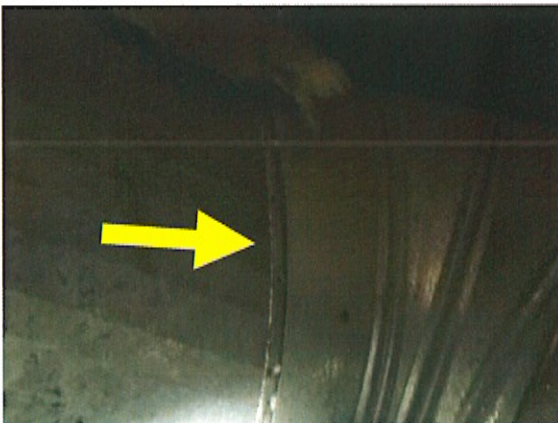
One of several locations where crawlspace air infiltrates the AHU ductwork
