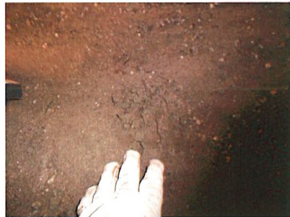
Wet/damp soils cover much of the crawlspace floor around both AHU's
