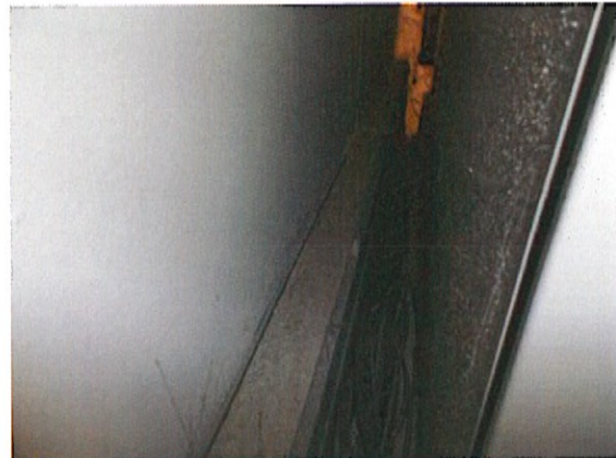
Poor housekeeping behind cubical sections up against the exterior wall areas
