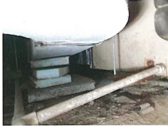
AHU's are in close proximity to damp crawl space soils
