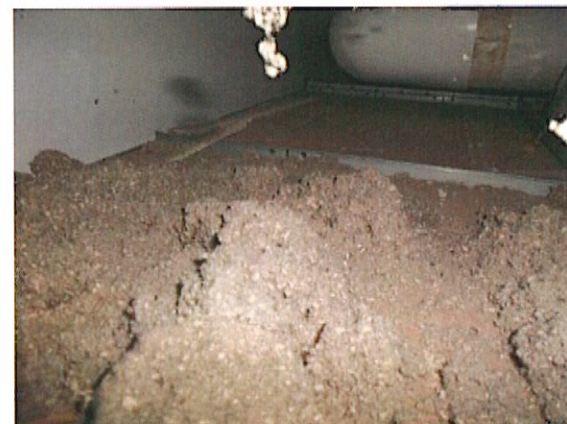
Rodent disturbed insulations on top ceiling of tile, visible signs of rodent urine and pipe condensation
