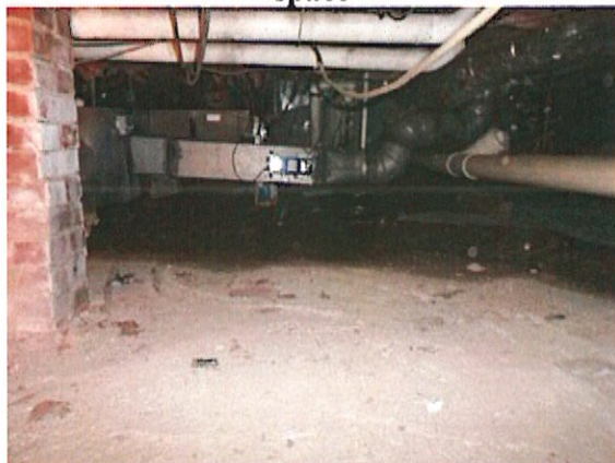
Settled damp soil covers the cement floor area at west end of crawlspace
