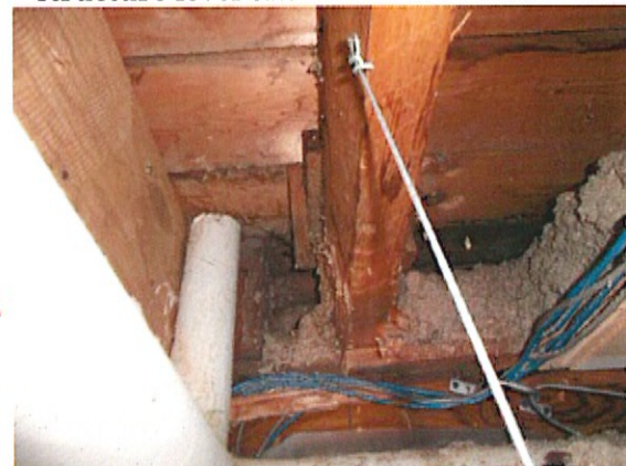
Above damaged ceiling tiles, disturbed cellulose insulations by rodent activity
