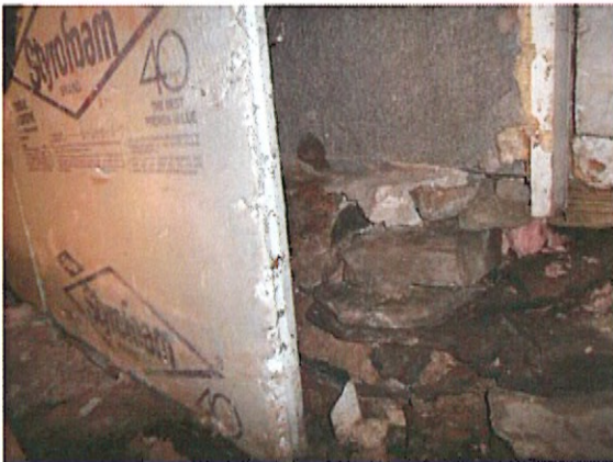
Conditions behind ridged foam board for crawlspace foundation walls
