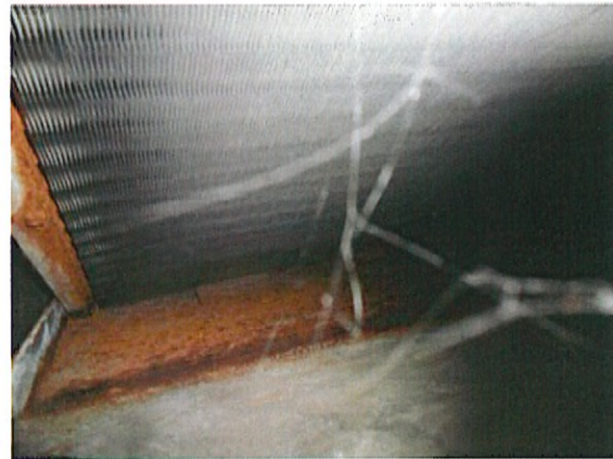
AHU's have significant rust for condensate pans
