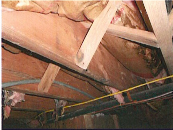
Floor joists appear to be in good shape, with many joists just starting to grow fungi
