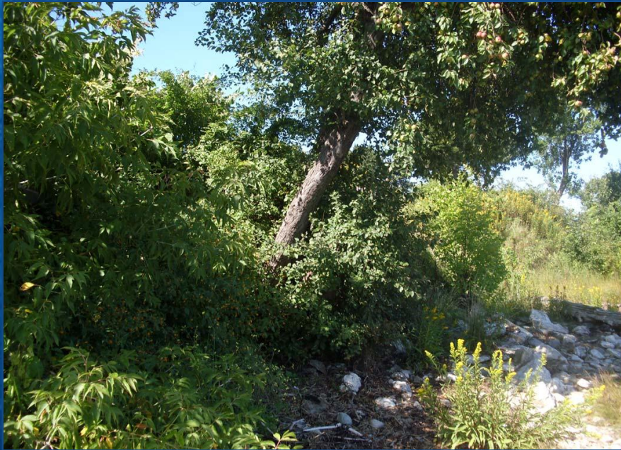
Block failure between Avon and McKinley.
