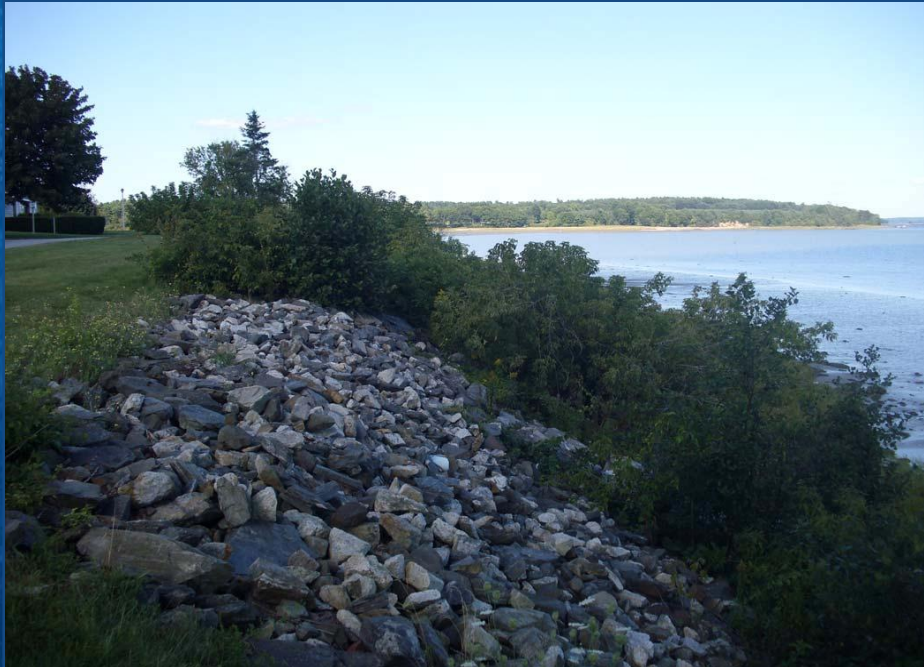
Poorly sorted rip-rap stabilization at McKinley.
