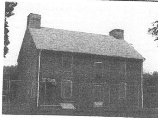
a. A view showing the exterior of the house in its mothballed condition.
