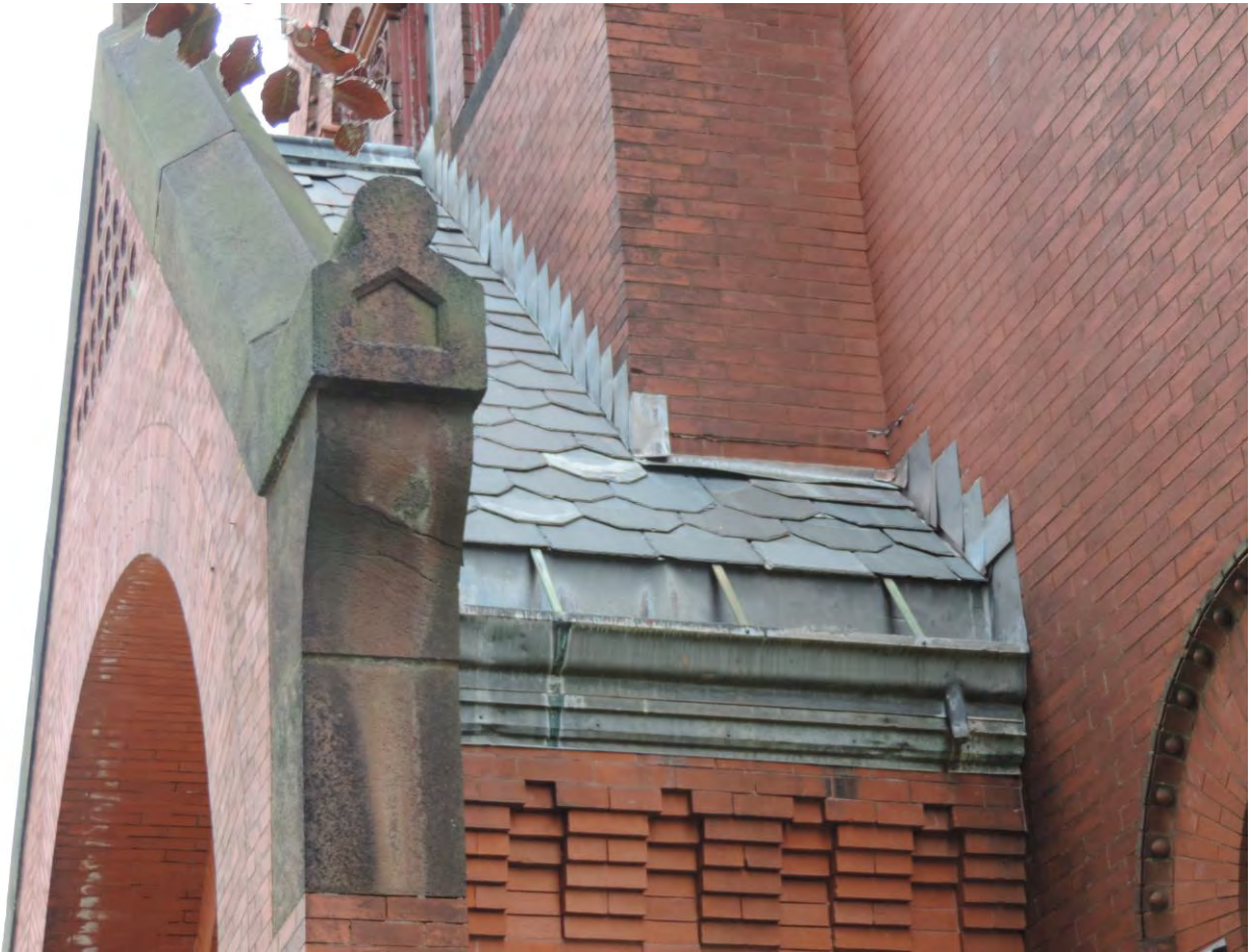
Rogers missing slates lifting flashing
