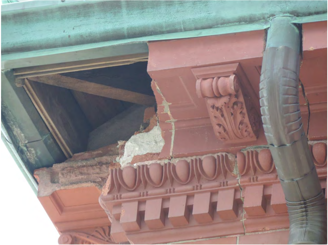
Oxford eave damage
