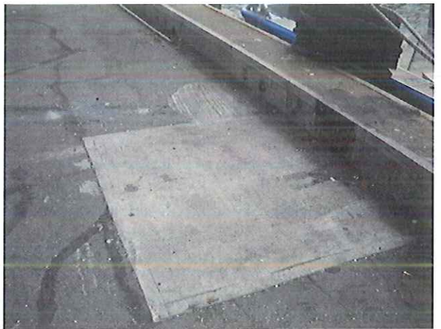
Concrete Patched Sink Hole
