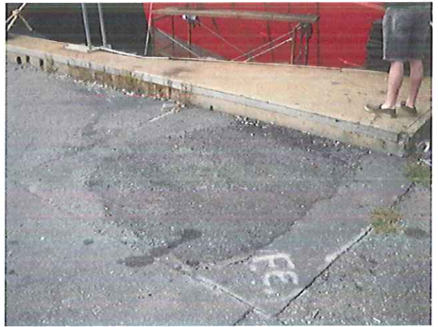
Asphalt Patched Sinkhole
