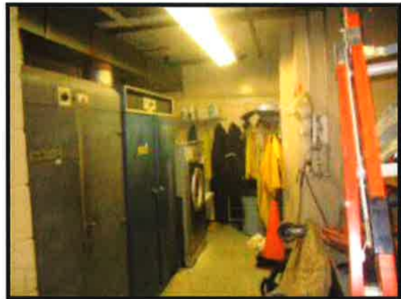
Station 1 Turnout Gear Room
