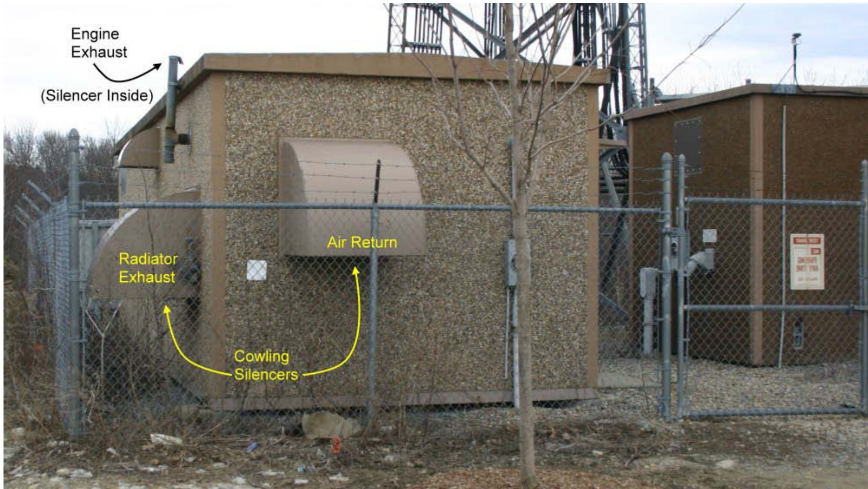
Figure A-2 Field Image of Equipment Shelters used by Verizon Wireless (with generator) and AT&T (on right)
