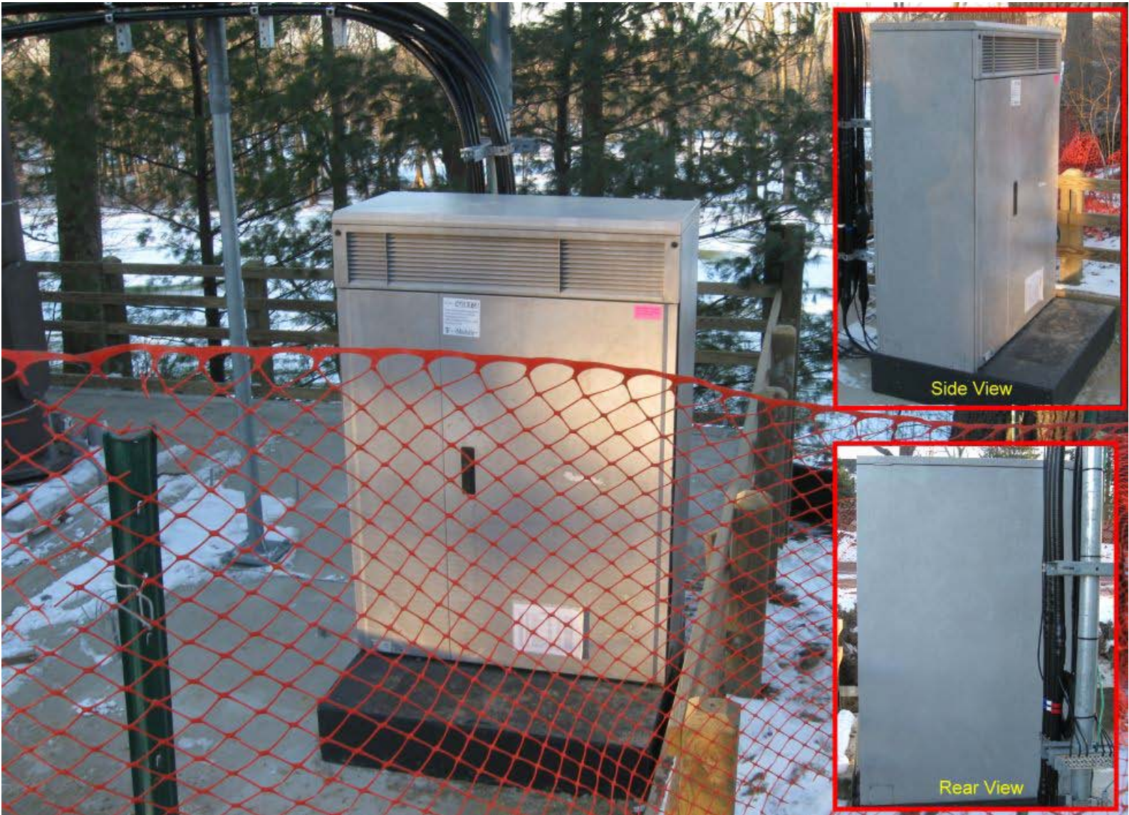
Figure A-3 Field Images of BTS Equipment used by T-Mobile. MetroPCS uses similar cabinets.
