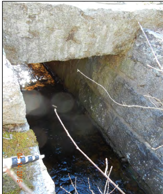
Photo No. 6 – Downstream railroad crossing – hydraulic outlet of south wetland (1,200 feet south of Kelsey Rd culvert)
