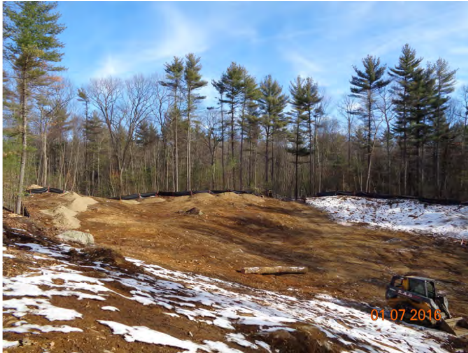
Photograph 3: Overview of Enhancement Area with top soil and vegetation removed, looking northeast.
