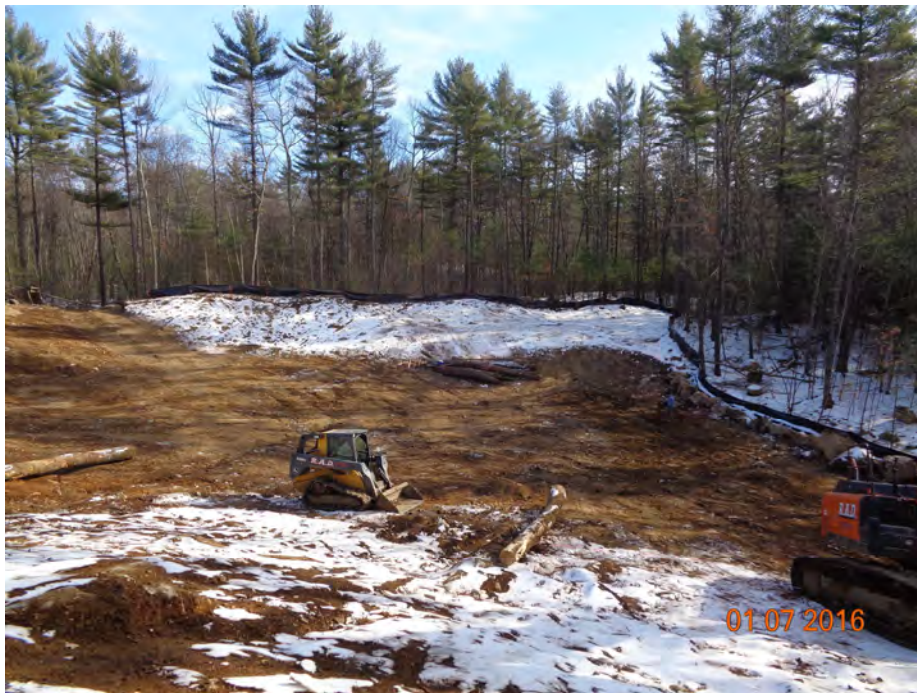
Photograph 4: Overview of Enhancement Area with top soil and vegetation removed, looking east.
