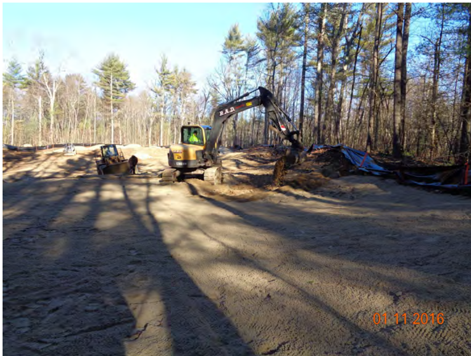
Photograph 6: Overview of Enhancement Area looking north while supplemental course material is added, looking northwest.
