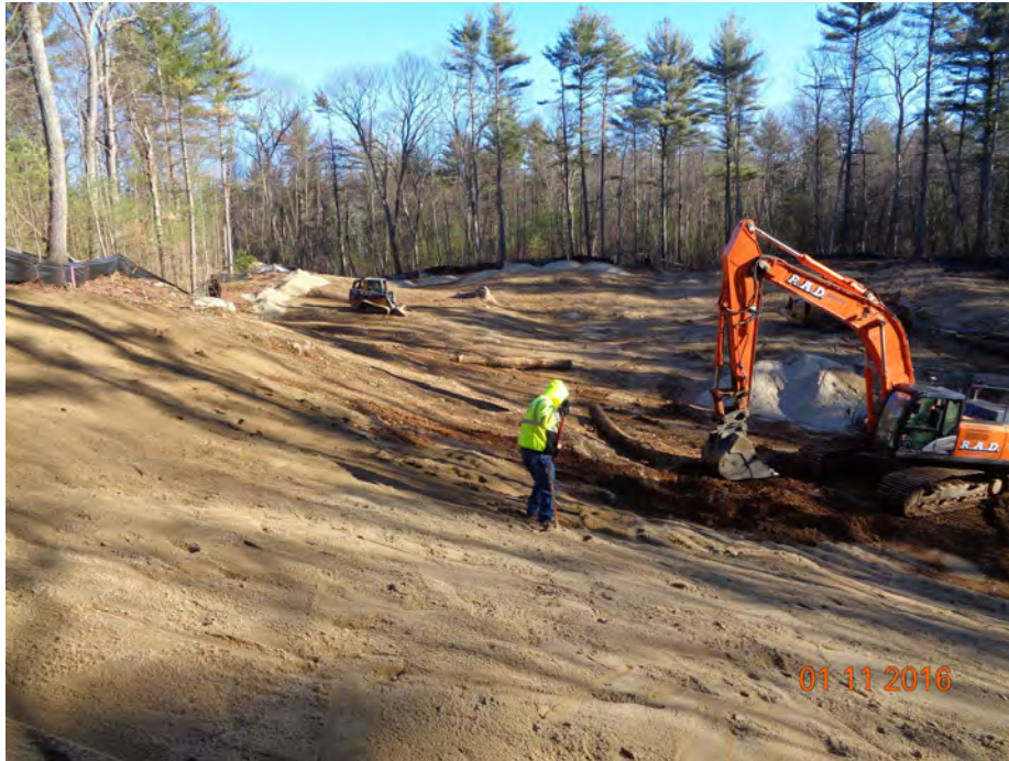
Photograph 5: Overview of Enhancement Area looking north while supplemental course material is added, looking northeast.
