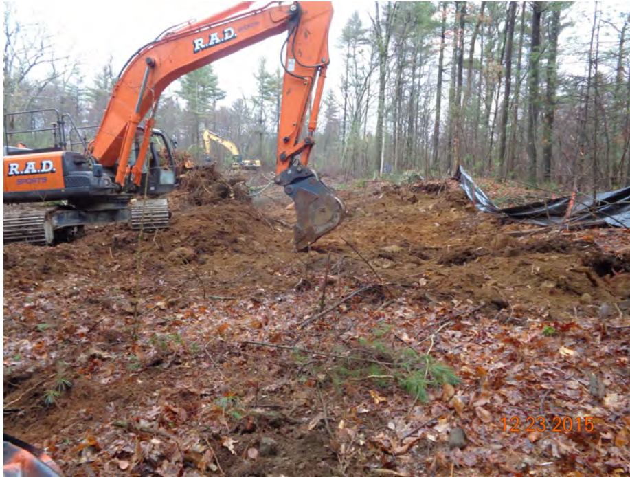
Photograph 1: Overview of Enhancement Area while top soil is being removed to expose native soil material.
