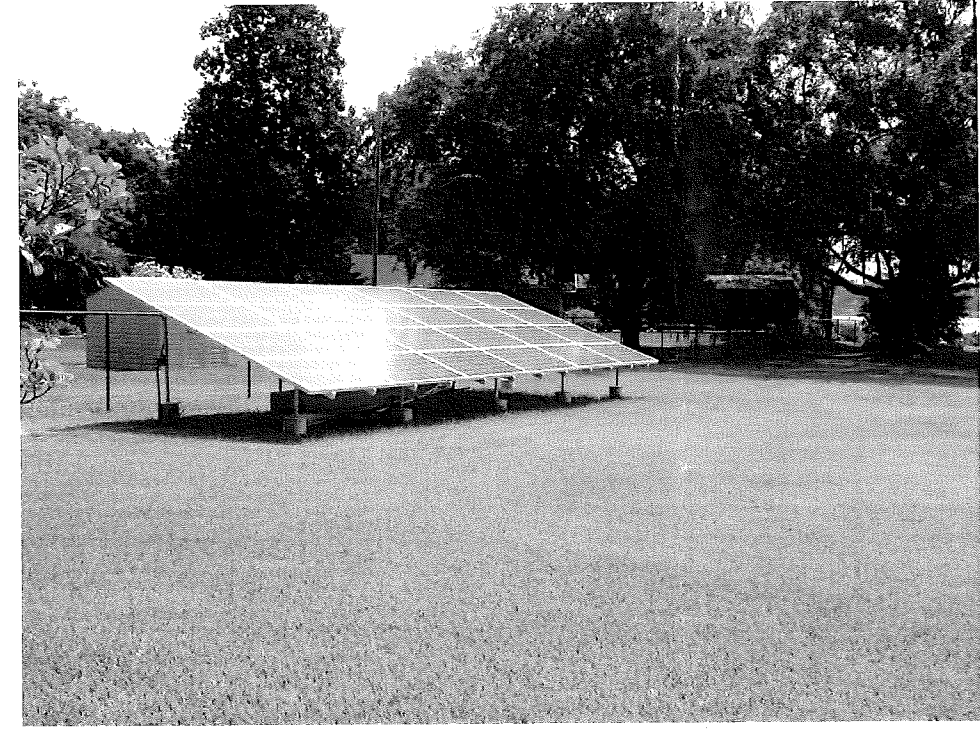
3 SIMILAR GROUND MOUNT ARRAY
