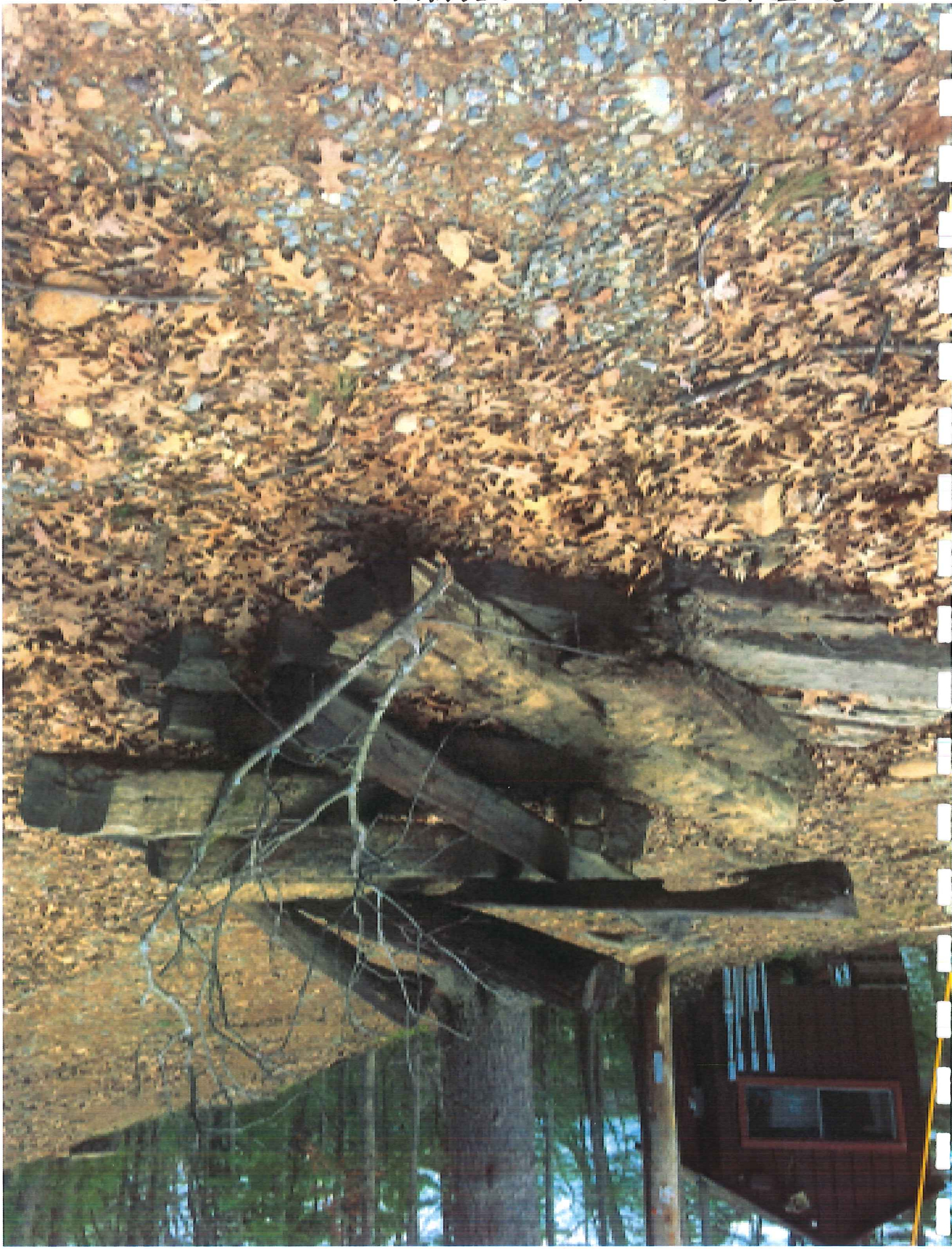
PHOTO #2 WOOD WALL REMAINS MAY 2015
