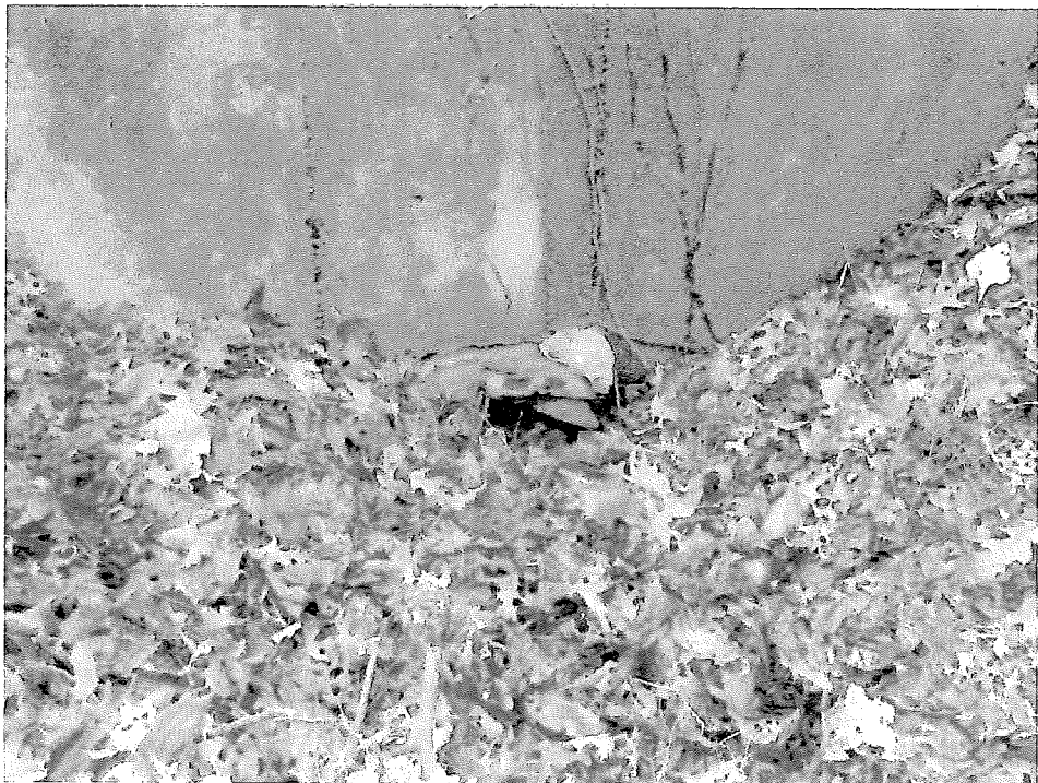
Photo D. View of the partially collapsed and clogged culvert below the headwall on the eastern side of Woodcrest Road. Photo by B. Prokop, November 25, 2014.
