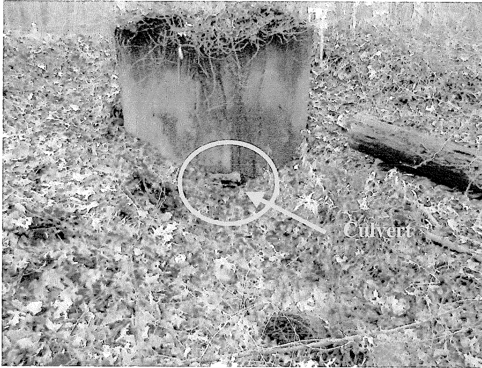
Photo C. View of the headwall on the east side of Woodcrest Road as seen from the wetland. Photo by B. Prokop, November 25, 2014.
