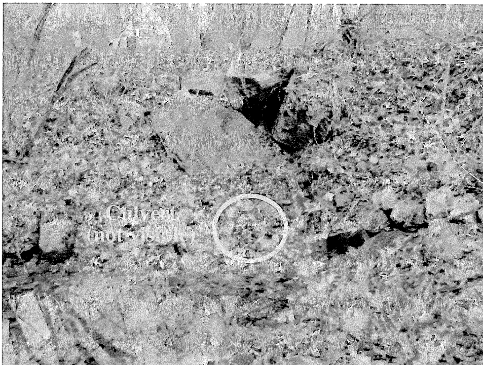
Photo F. View of the western side (inlet) of the Woodcrest Road culvert replacement showing the existing riprap. Culvert proposed for replacement is buried in sediment at the bottom of the riprap and not visible. Photo by B. Prokop, November 25, 2014.
