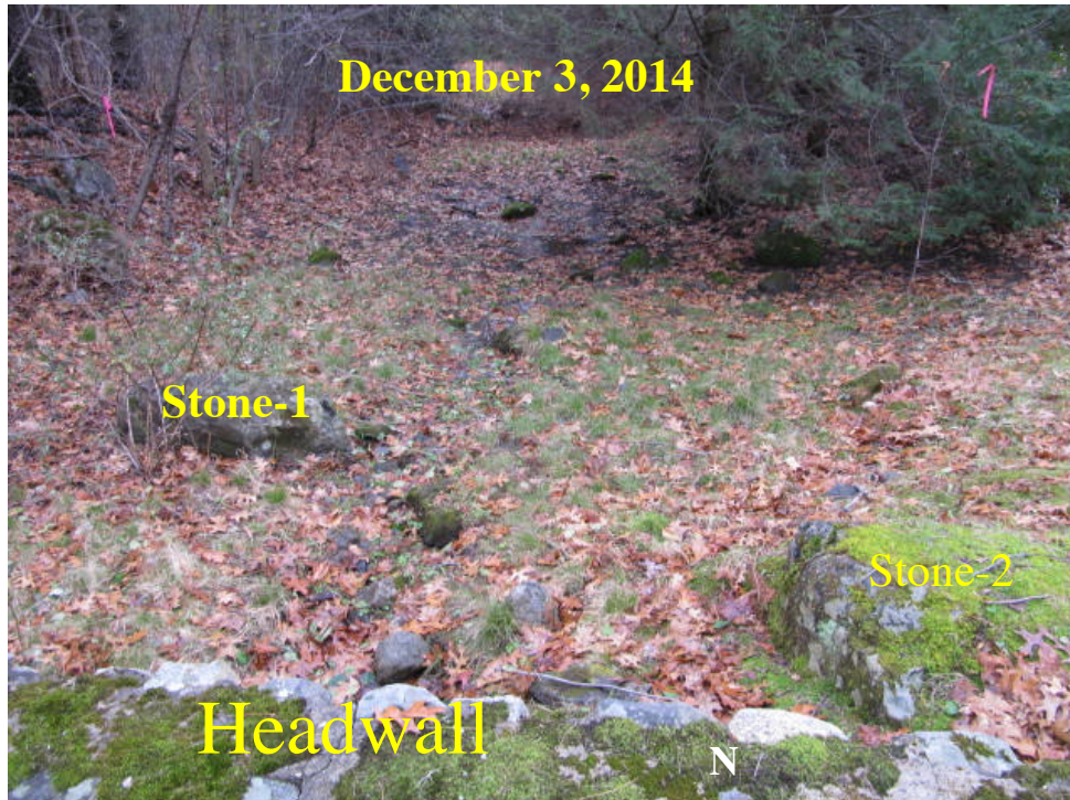
Photo A. View of the downslope (outlet) side of the culvert at 49 Woodcrest Road in early winter 2014. Photo by B. Prokop.
