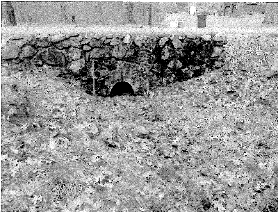
Photo D. View of the outlet side of the culvert between 48 - 49 Woodcrest Road. Photo by B. Prokop, November 25, 2014.
