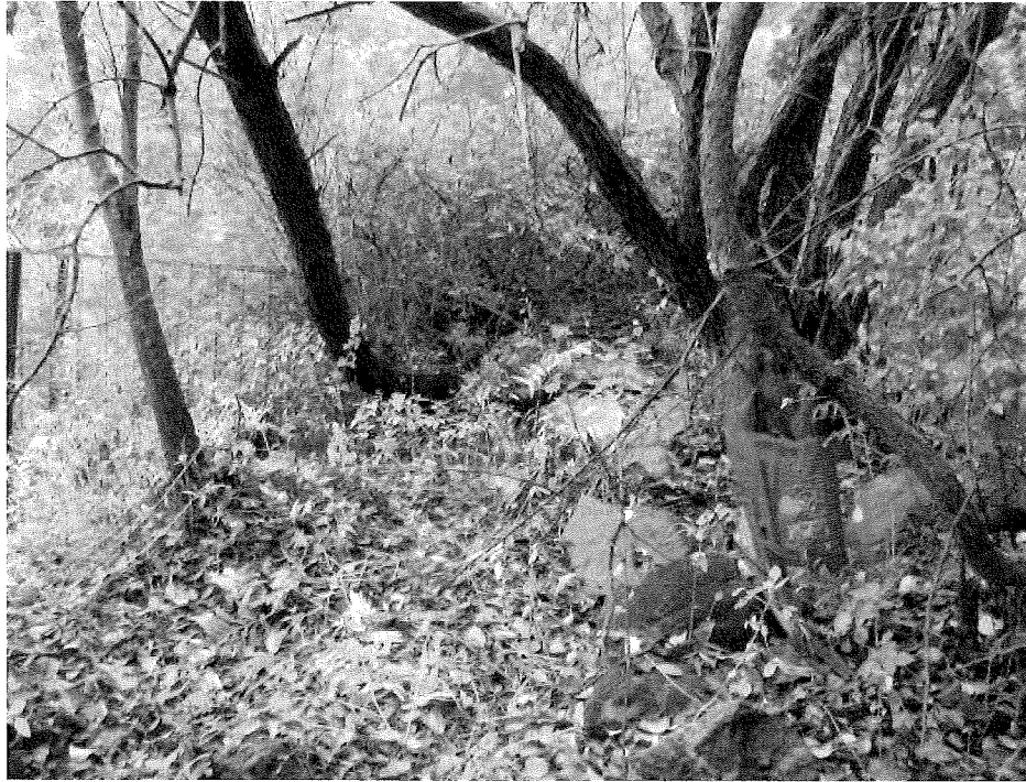
Photo C. View of the rock debris and the various trees on the inlet side of the culvert that need to be removed. Photo by B. Prokop, October 2, 2014.
