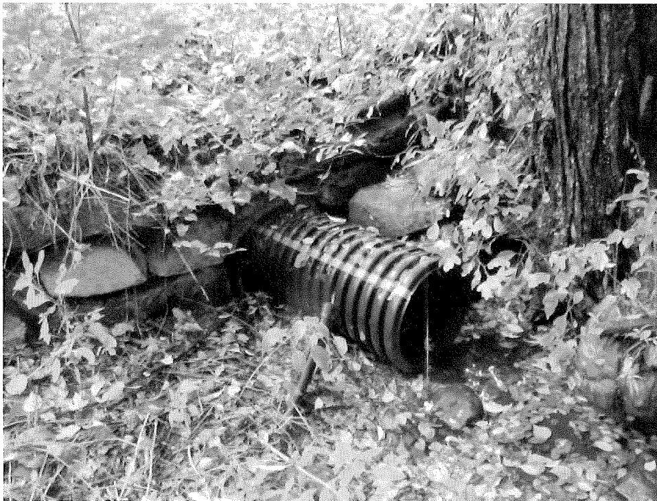
Photo D. View of the plastic pipe insert and rock headwall on the outlet side of the road. Photo by B. Prokop, October 2, 2014.
