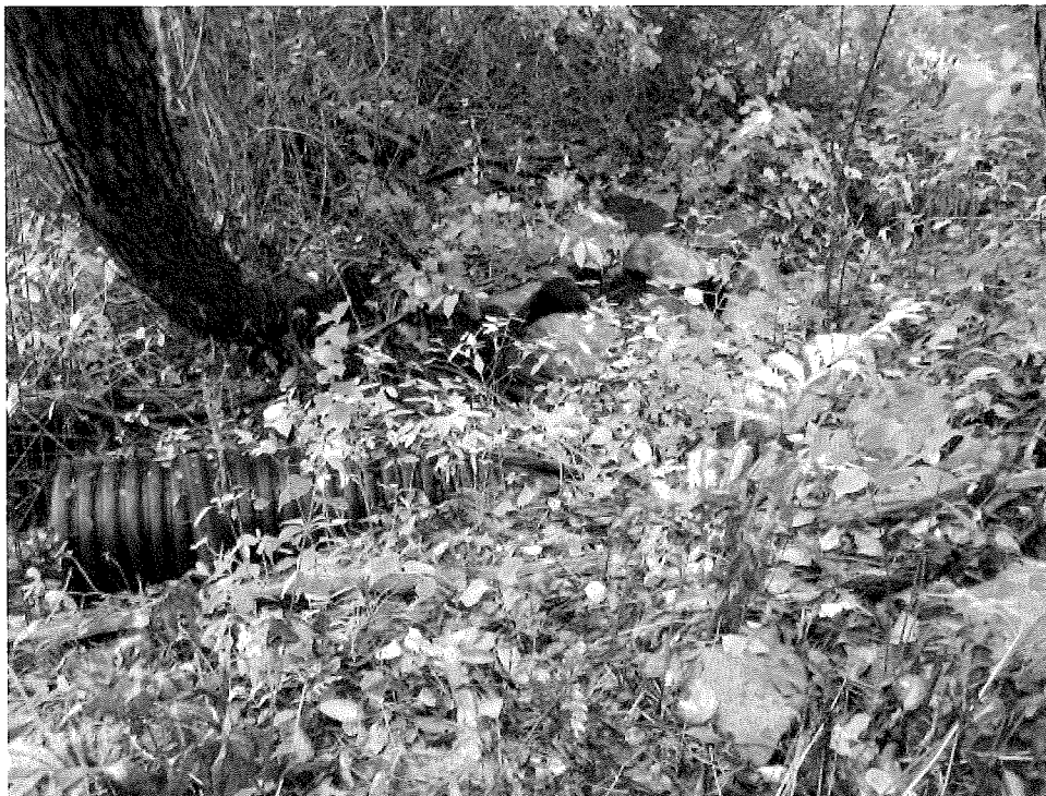
Photo B. View of the northern side (inlet) of Kelsey Road showing the 15" plastic pipe insert. Photo by B. Prokop, October 2, 2014.
