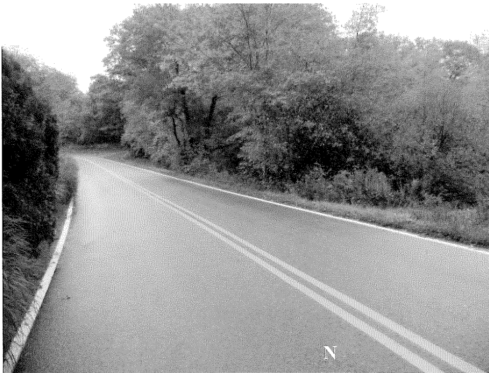
Photo A. Northerly view of Kelsey Road where the culvert will be replaced. Photo by B. Prokop, October 2, 2014.
